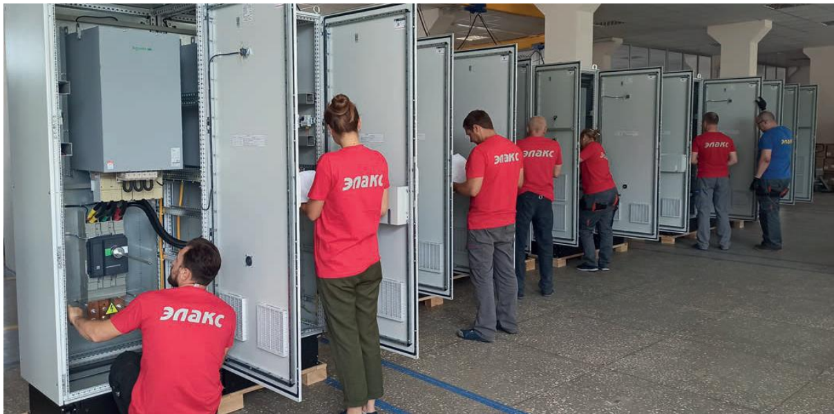
ELAKS is a biggest panel builder in electrical engineering in Ukraine. They have relocated a part of facilities in Bratislava on March 2022.
