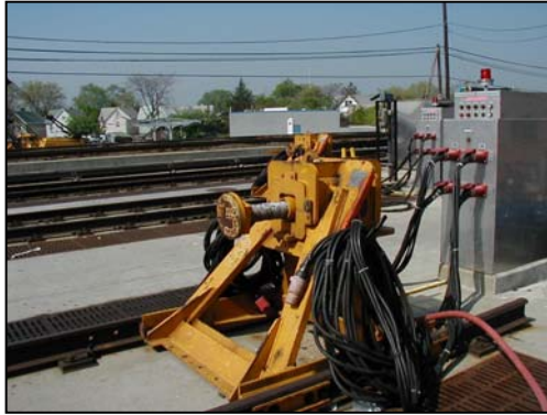
(20) Bumping Post with Hydraulic Ram
