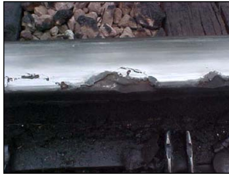
Shelly Spots on Gage Side of Rail Head
