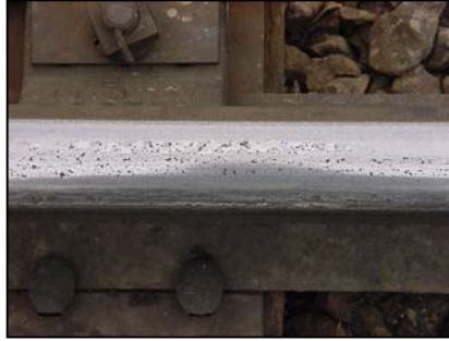
Section of Rail Showing Flaking
