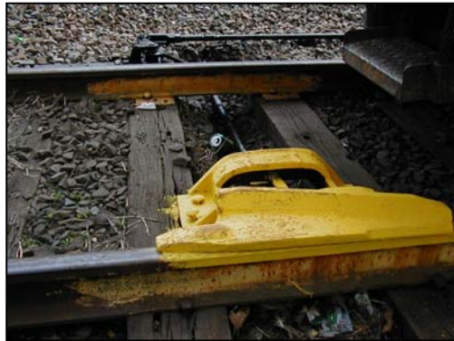
(21) Sliding Block Derail
