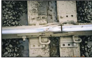
Deficient Rail Fastening System (Caused by Foul Ballast)
