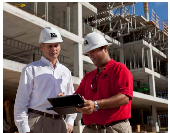
Kaufman Lynn Project Manager and Superintendent working off of Procore on their iPad on the jobsite.
