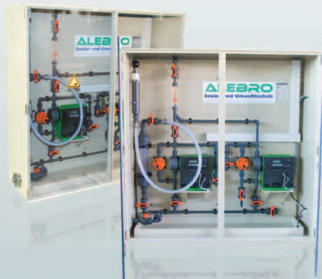
Dosing system installed in cabinet
