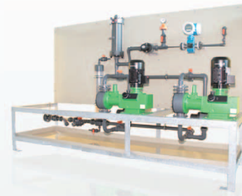
Sodium hypochlorite dosing station
