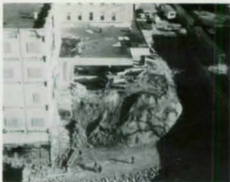
Fig. 3. Demolition of main entrance and preparation of 5-story existing structure for steel tower.
