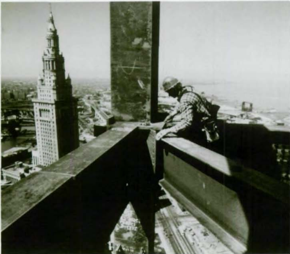
High on 38th floor, worker erects steel frame. Historic Terminal Tower is in background. Kodiak cranes (r.) were designed especially for project. Four-story crane base fits in elevator shaft.
