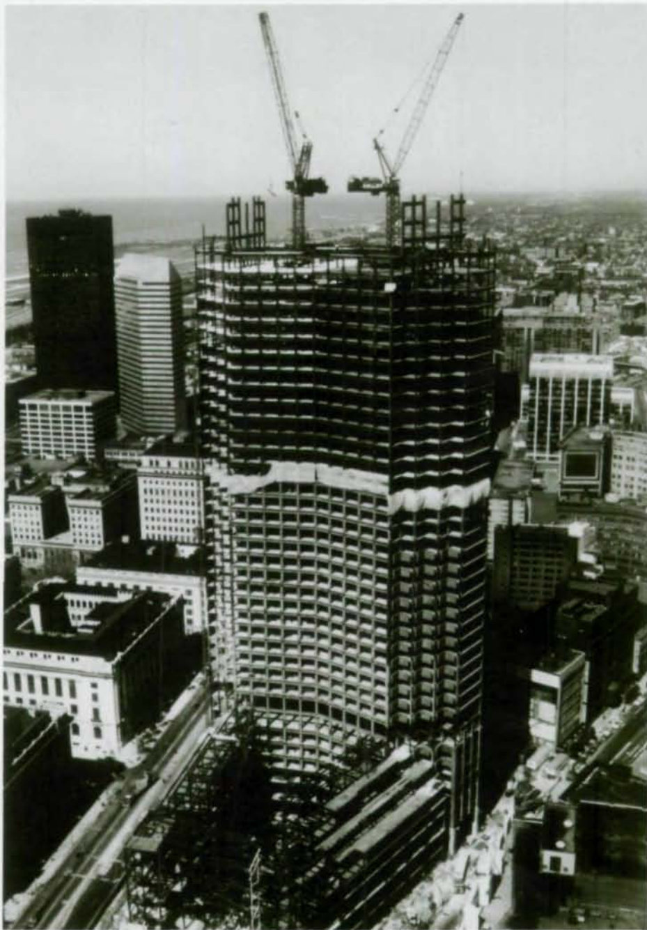
Structural steel tower of Sohio Building rises in Public Square area. More than 20,000 tons of steel went into tower and atrium (foreground). Rendering of atrium above, r.
