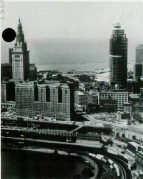
Aerial of Public Square area of downtown. Last steel erected June 22, 1984, with early occupancy slated for Spring, 1985.
