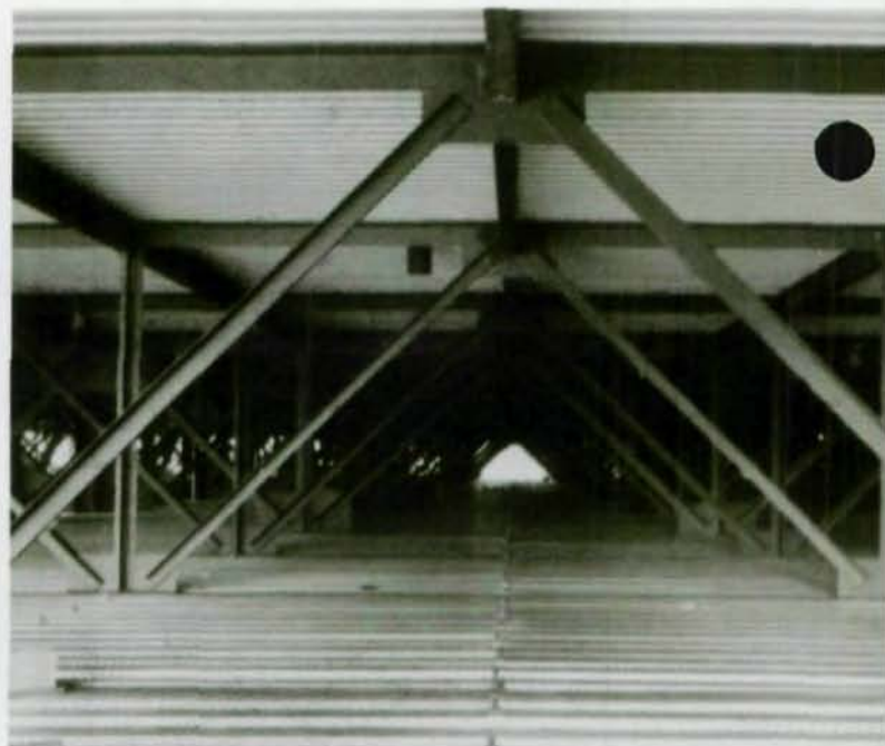
View of interstitial framing and extended 2-bed patient rooms (l.). Closeup (above) of interstitial space before deck pouring. Photos courtesy Albert Kahn Associates. Below, r.: interstitial truss swings into place. Inpatient bed floors beyond. Photo courtesy Barton/Malow.
