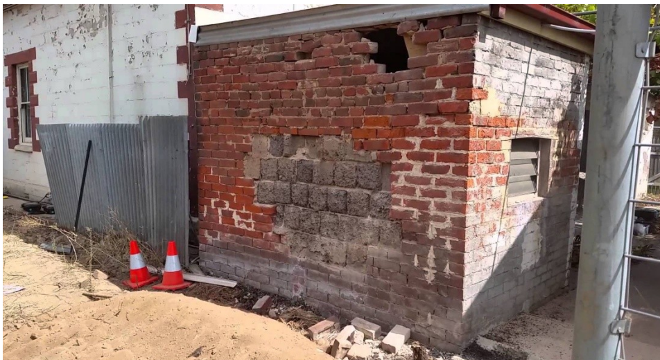
Figure1.4: Observing building vibration damage caused by an 18t pad foot roller ( www.youtube.com/watch?v=acBaXbMHNfE )
