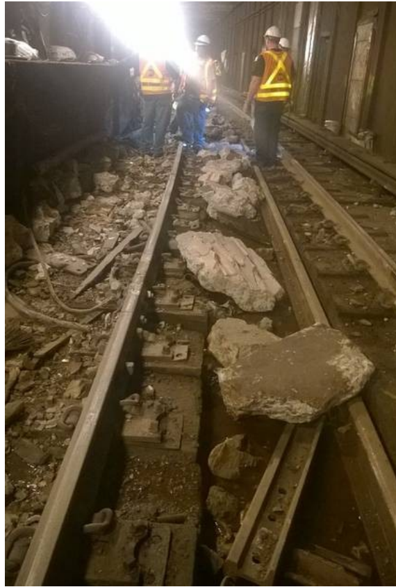
Figure 1.5: Subway Train Derails in Brooklyn Bench walls and concrete tunnel linings are susceptible to age, water damage and vibration from construction above.
