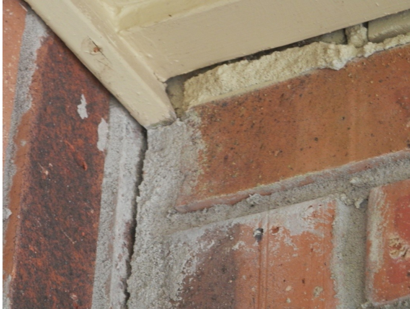
Figure 5.5: Damage in plaster due to road construction, recent insurance adjustment claim for a home damaged by construction next door, Florida, USA. ( www.toddclaimservice.com )
