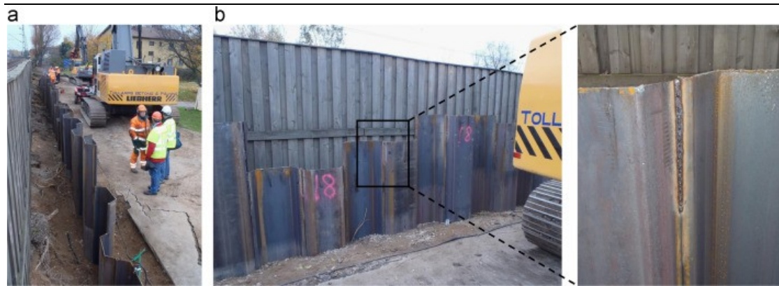
Figure 6.5: Installation of the sheet pile wall: (a) general view after installation of sheet piles up to a depth of 10=16 m with the small rig, (b) welding of the top 0.3 m, adapted from Dijkmans et al (2016).
