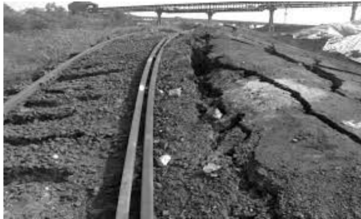
Figure 3.23: The effect o soil heave on the facilities (railway lines) after Reddy et al (2008).
