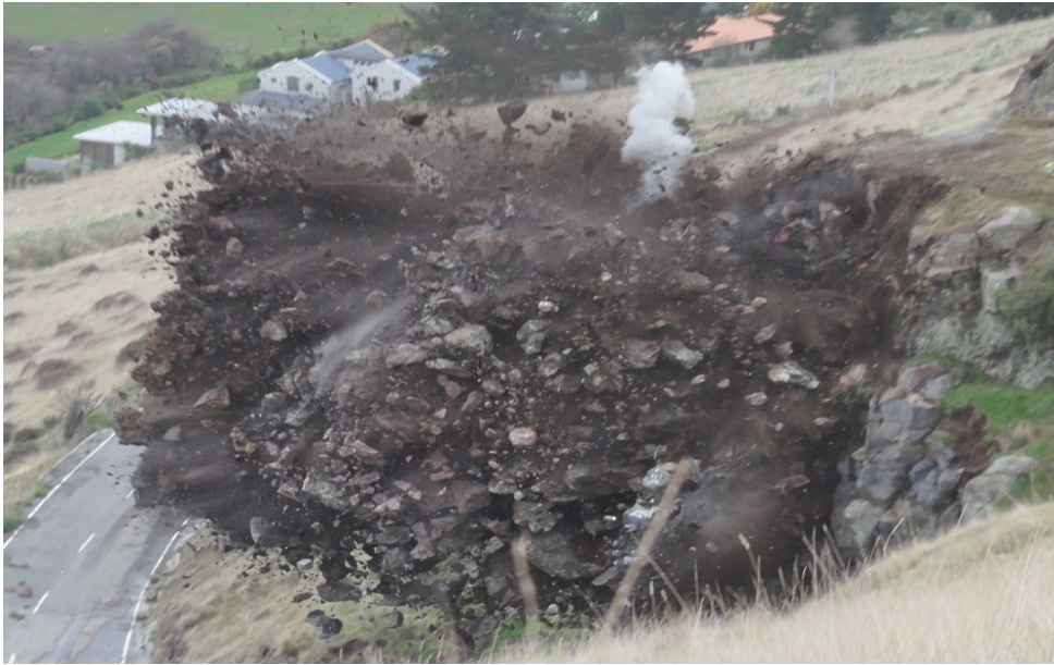
Figure 1.10: Blasting for securing roads, Evans Pass Rd, Sumner, Christchurch Date: July & August 2012, ( www.abseilaccess.co.nz )
