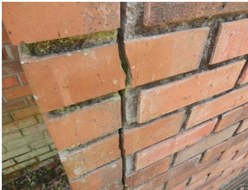
Figure 5.6: Damage in wall due to road construction, recent insurance adjustment claim for a home damaged by construction next door, Florida, USA. ( www.toddclaimservice.com )
