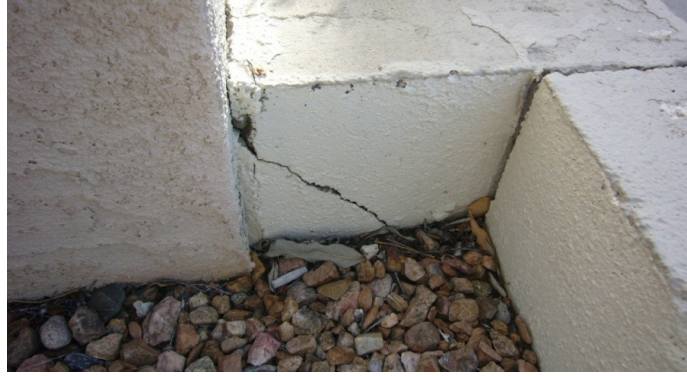
Figure 5.2: Cracks in exterior property wall, ( http://vibrationdamage.com/understanding_vibration_damage.htm ).
