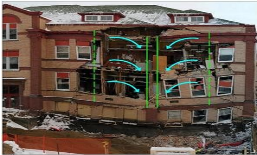
Figure.1.1: Collapsing of Minard Hall facade along the northwest wall of the building due to excavation and near the excavation site, piles been driven (after Nowatzki 2009)
