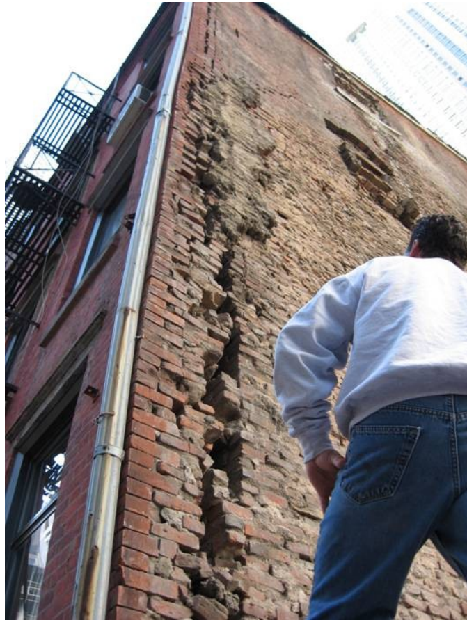
Figure1.3: Damage due to construction vibration ( www.exponent.com )
