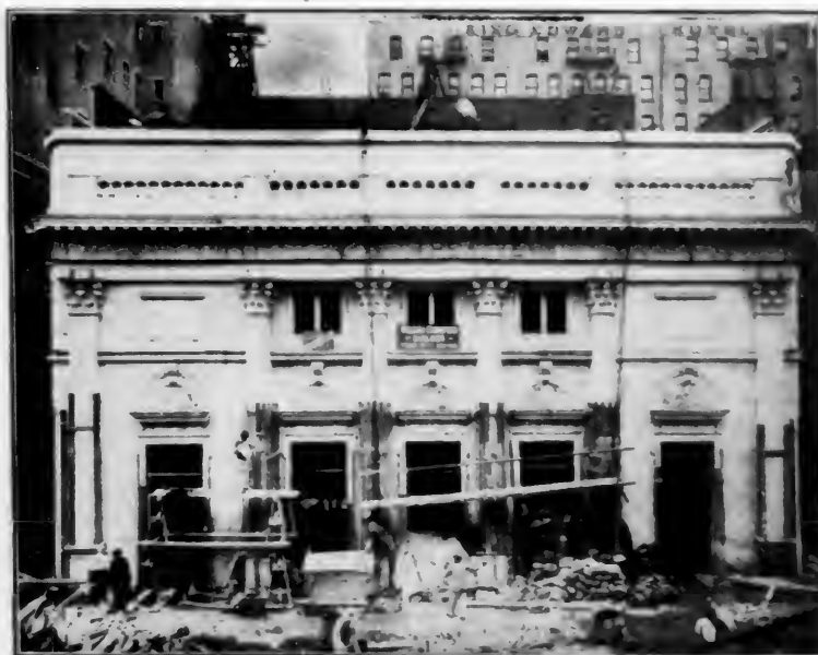
New Cort Theatre under construction in 48th Street, just east of Broadway, New York City.
