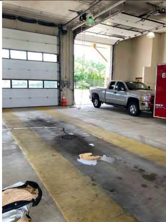
Description Floor drain with oil-water separator manhole on background Viewing Location/Direction Fire fighting building garage, looking southwest
