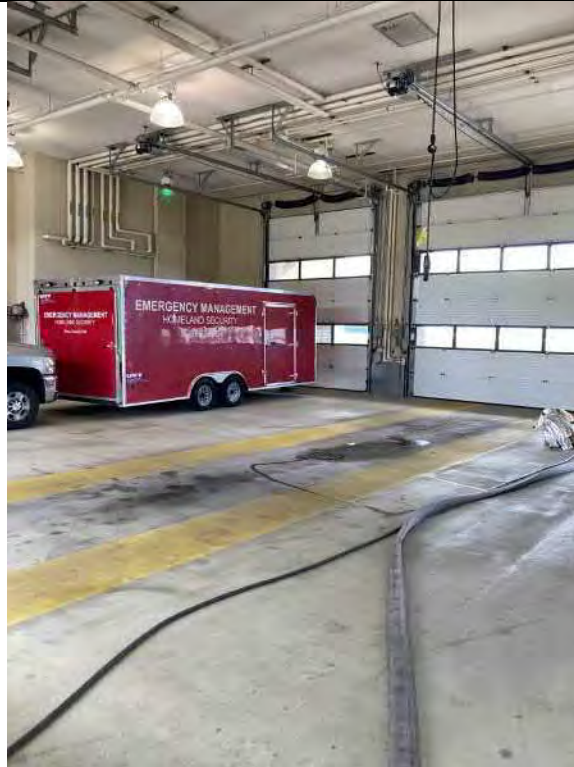
Description Typical view of garage bay, floor drain in center with staining Viewing Location/Direction Looking northwest
