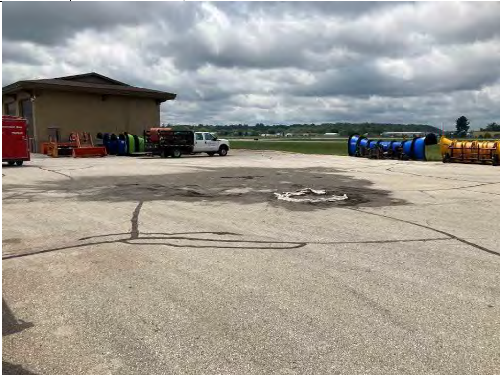
Description AFFF spill around storm drain Viewing Location/Direction West side of building
