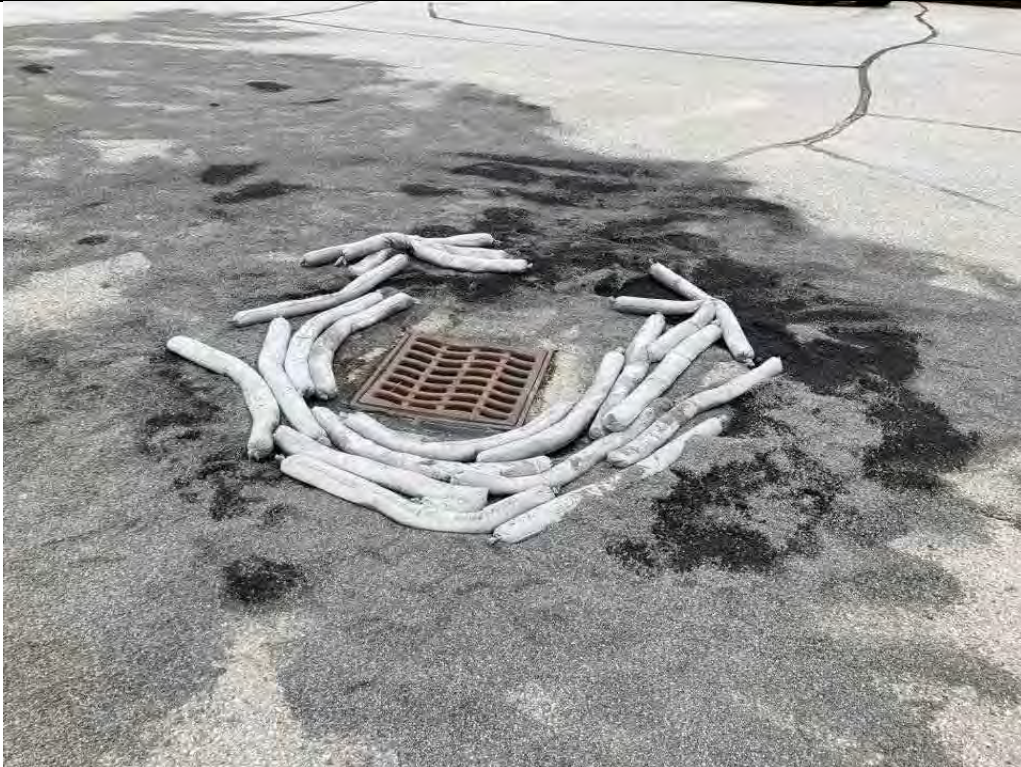
Description AFFF spill containment around catch basin Viewing Location/Direction West side of building
