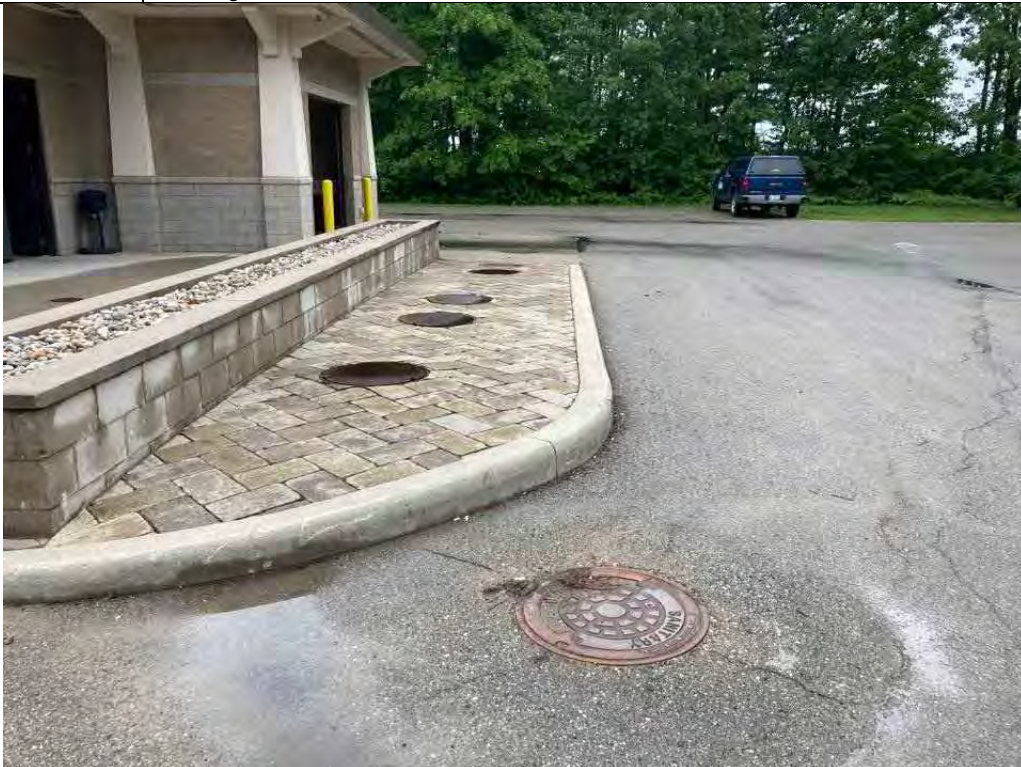
Description Underground rinseate tanks adjacent to sanitary sewer Viewing Location/Direction Tanks and sewer manholes in north side of building, looking west
