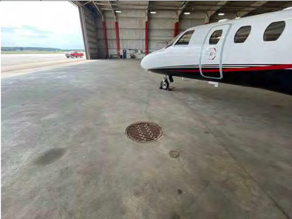
Description Storm drain near southwest corner Viewing Location/Direction Northwest corner facing West
