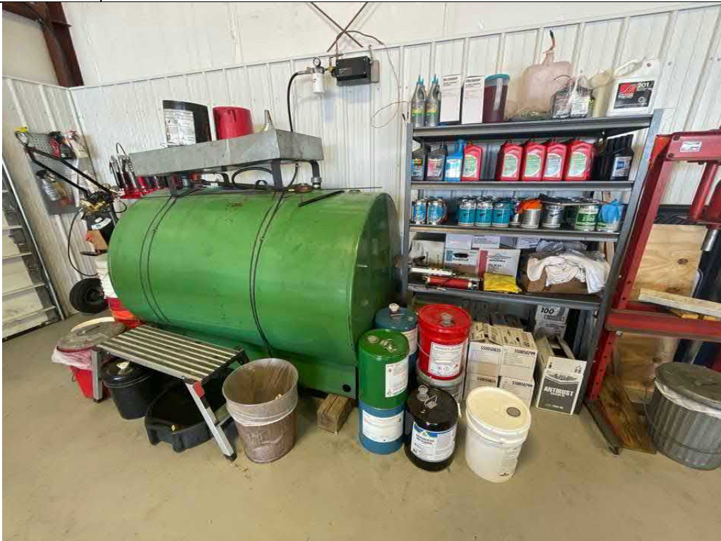
Description Used Oil AST and petroleum product storage Viewing Location/Direction Northeast corner
