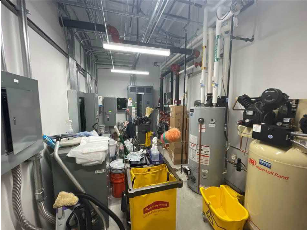
Description Utility room Viewing Location/Direction Central building
