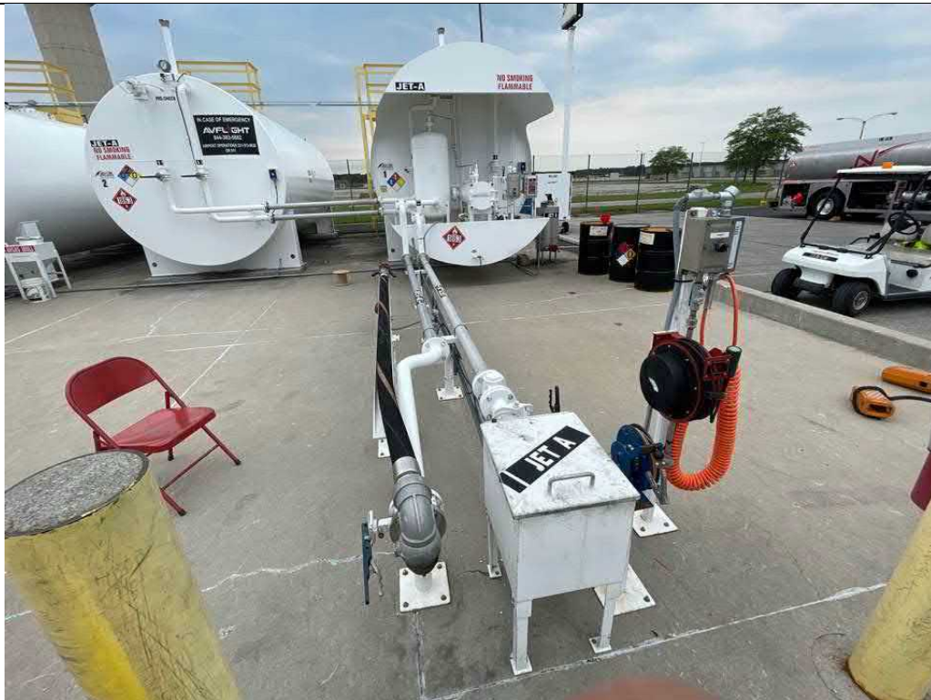
Description Fuel pump and lines - west
