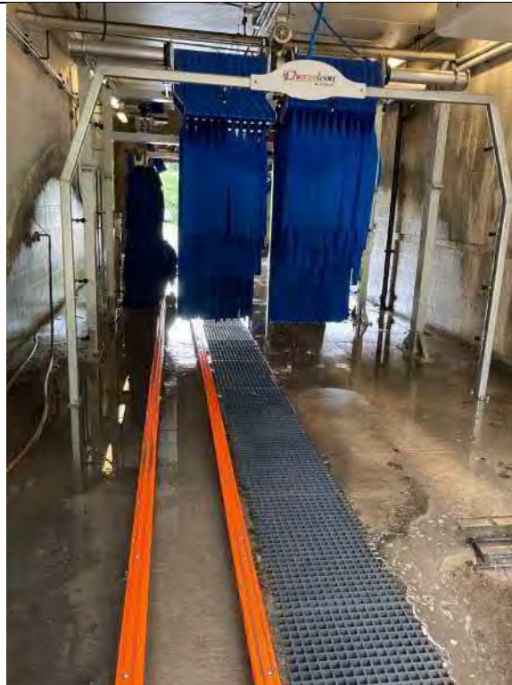
Description Car wash service bay with floor drains Viewing Location/Direction Looking south
