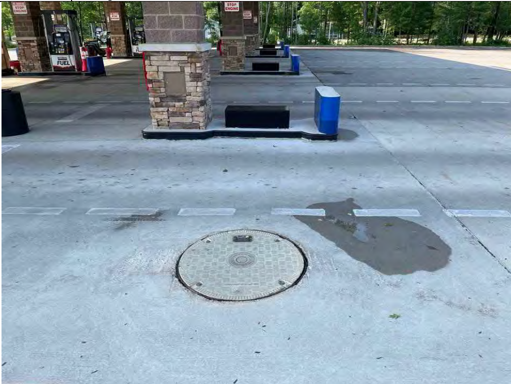
Description Underground storage tank for gasoline pumps Viewing Location/Direction Facing south
