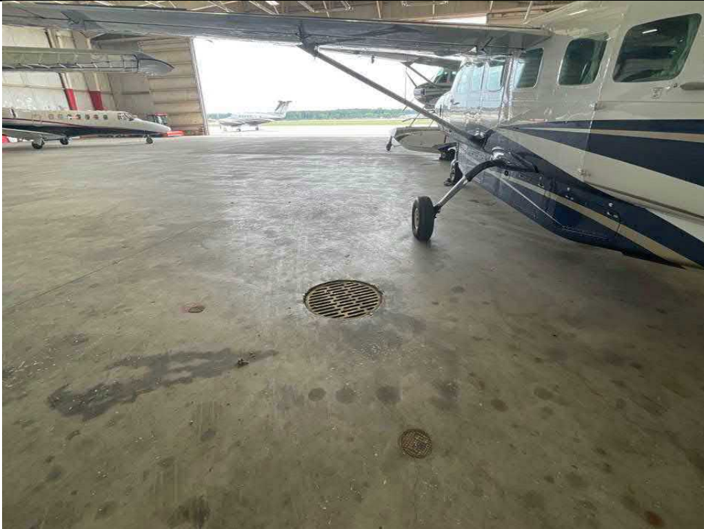
Description Storm drain near northwest corner Viewing Location/Direction Northwest corner facing southeast
