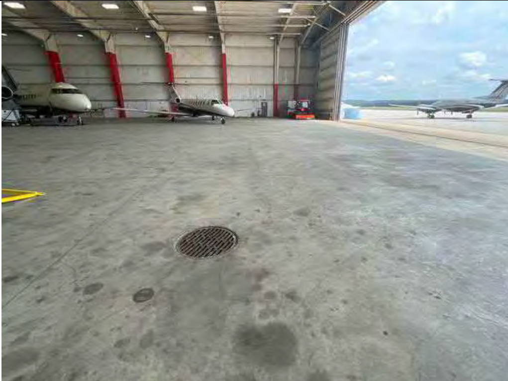
Description Storm drain near southwest corner Viewing Location/Direction Southwest corner facing east
