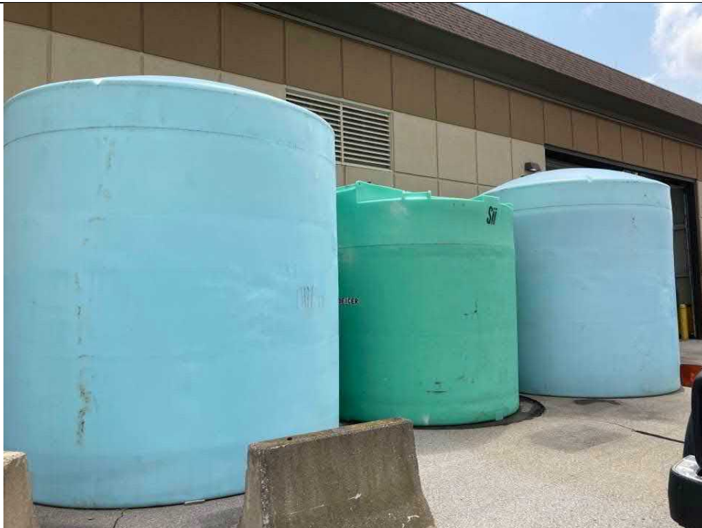
Description Storage tanks for deicer Viewing Location/Direction West side of building
