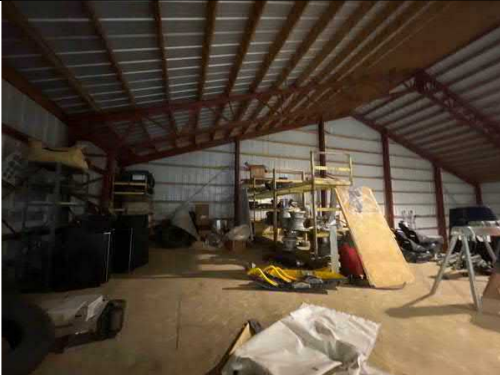
Description Upstairs storage in northwest corner Viewing Location/Direction Northwest corner facing north
