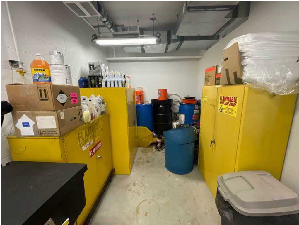
Description Hazardous chemical storage room Viewing Location/Direction North side of hangars
