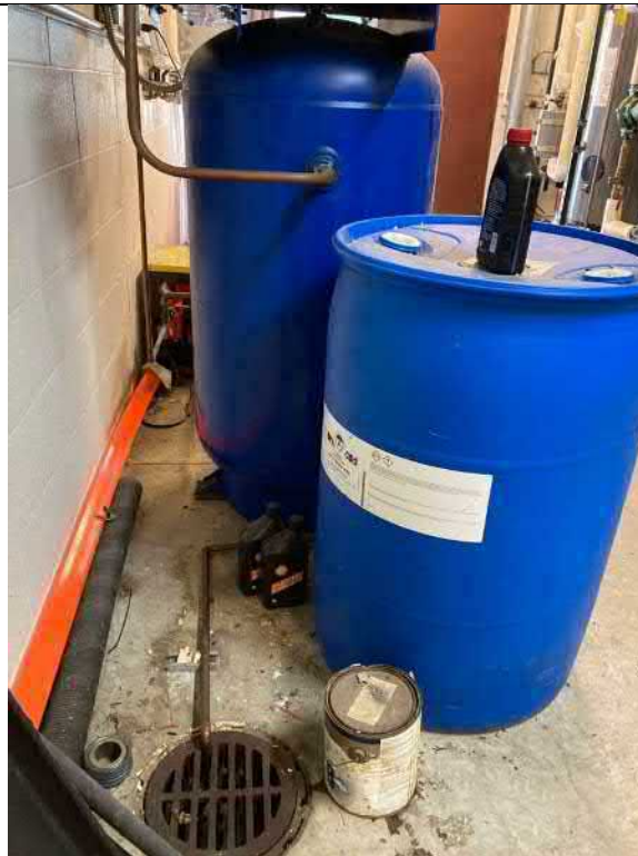
Description Compressor, condensate line to floor drain, drum with wax Viewing Location/Direction Operations room
