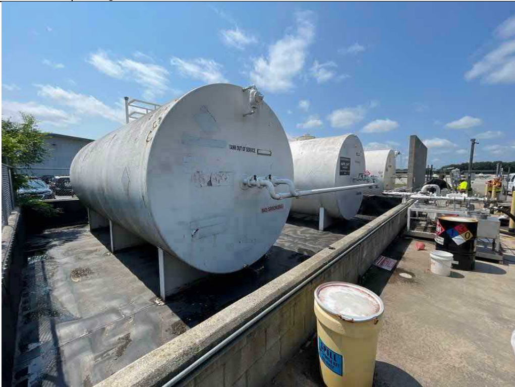
Description Fuel tanks in containment with liner system Viewing Location/Direction Facing southwest
