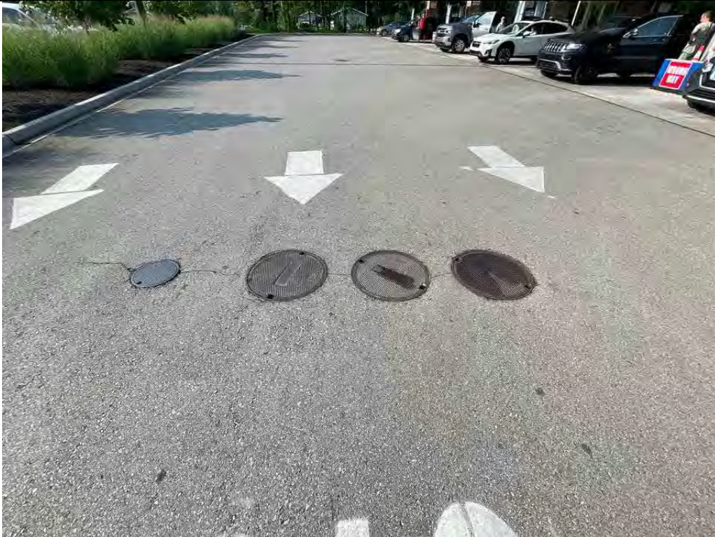
Description Manhole for waterline/storage tanks in northeast corner Viewing Location/Direction Facing south
