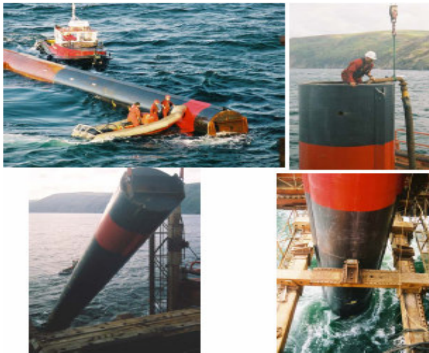
Figure 2.4 Installation of the monopile for the Seaflo marine current turbine off Foreland Point near Lynmouth
