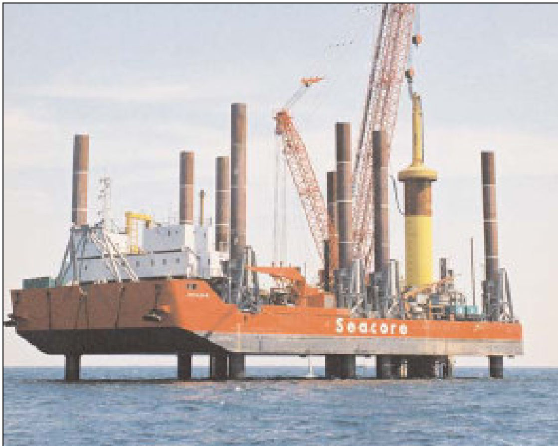
Figure 2.3 Seacore’s “Excalibur” jack-up barge which is most likely to be used in the installation of the marine current turbine
