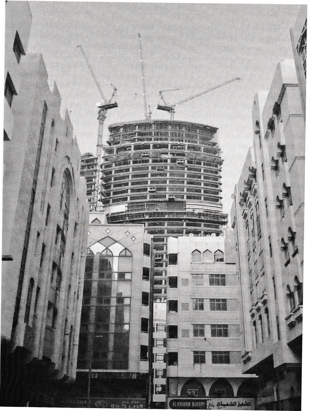
Old versus new in downtown Abu Dhabi. Pictured are closely packed 1970s-era buildings and one of their newer counterparts.
