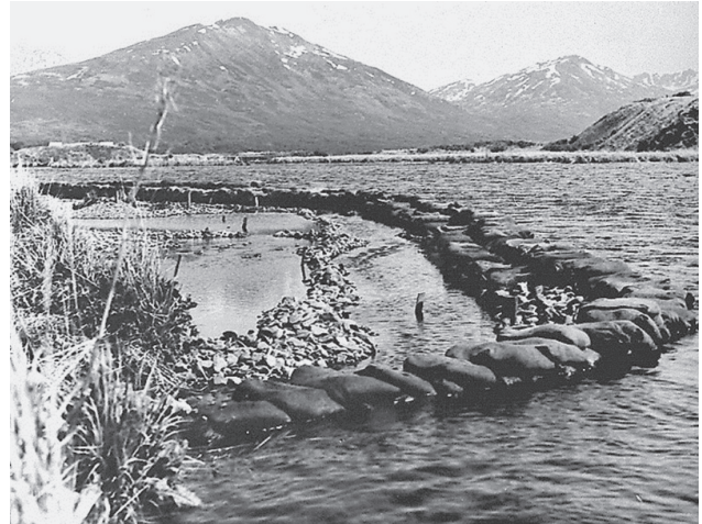
Coffer dam for construction of a two-way permanent salmon counting weir, upper Karluk River, June 1949. (Richard F. Shuman, Auke Bay Laboratory, Auke Bay, AK)
