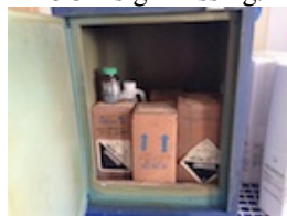
Old disintegrating boxes of acids in unvented acid cabinet.
