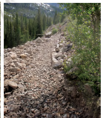
Before and after: clearing the trail and providing rock base (by breaking apart rocks and boulders) for the trail helps prevent erosion.
