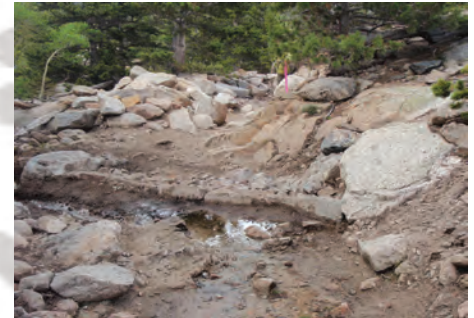
While not glamorous, creating water bars is essential trail work needed to prevent erosion on the trail.
