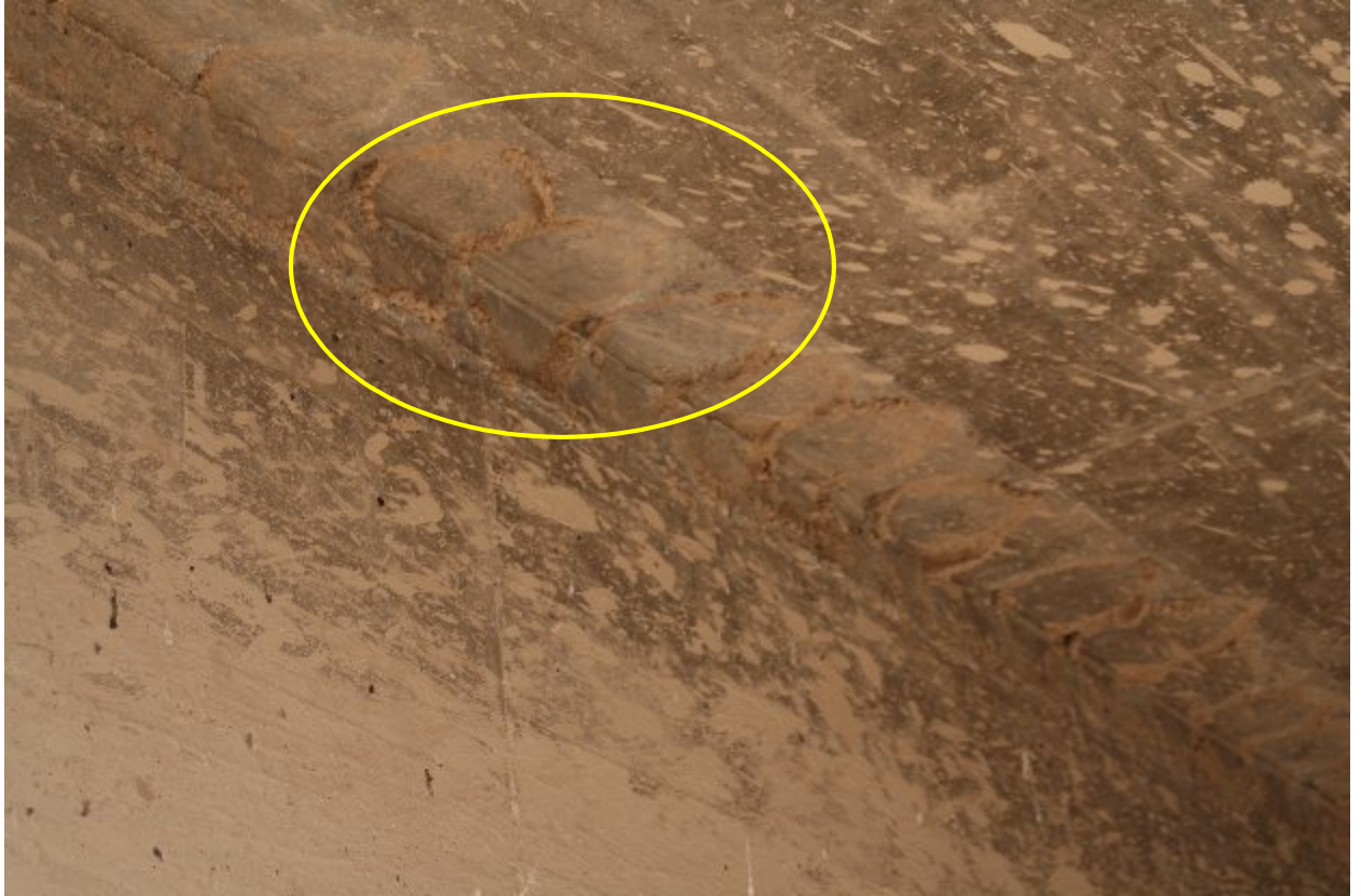
Photo 7. Evidence of previous swallow use of the eastern most box culvert for nesting. The yellow circle highlights locations of old nests placed against the culvert wall and ceiling.
