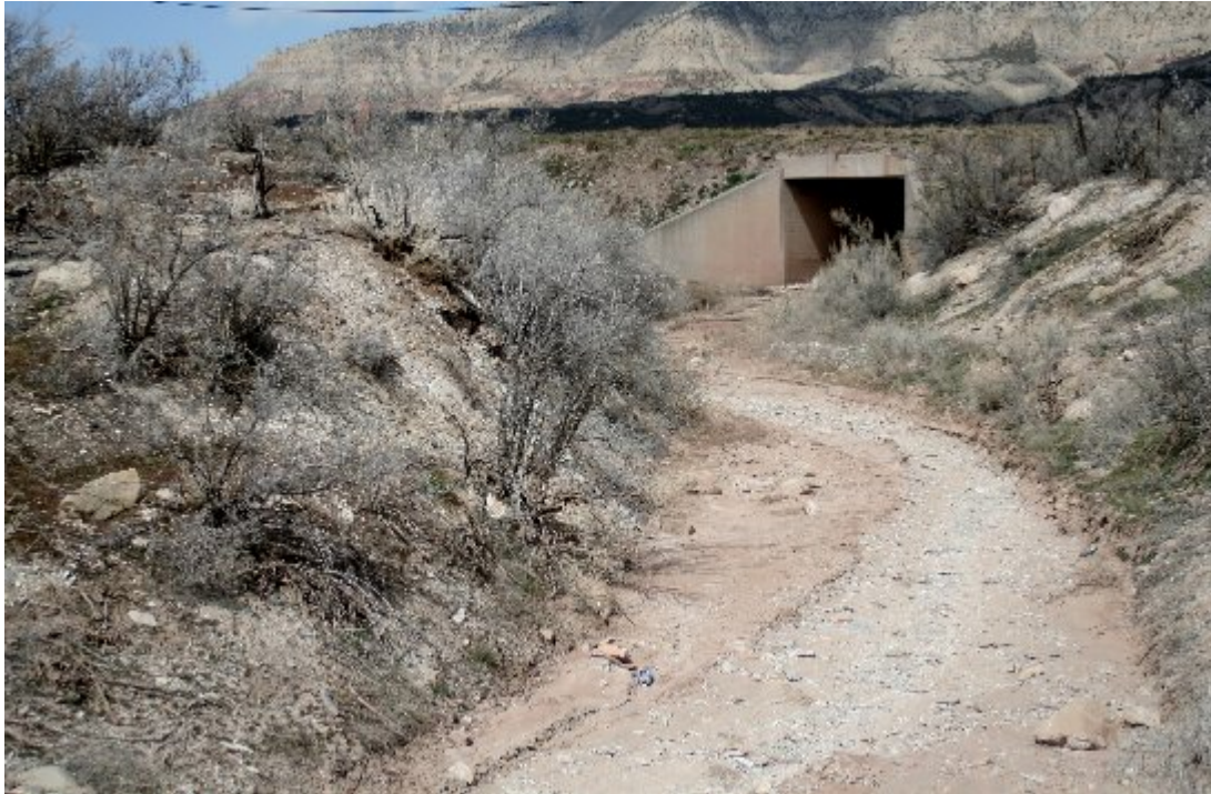
Photo 3. View north toward downstream side of eastern most box culvert on the 20 acre parcel.
