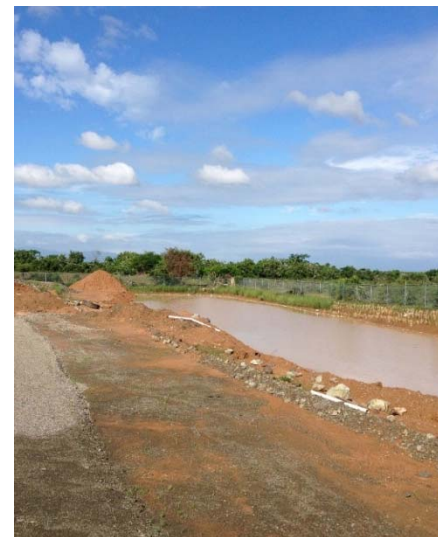
Figure 1-2. Standing Water present in the Stormwater Pond
