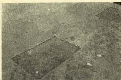
FIG. 4.—A patched area in a pavement filled to top with binder is being allowed to compact under traffic before top course is placed.
