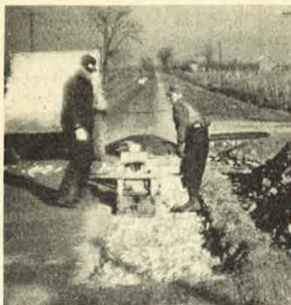
FIG. 1.—Compacting base aggregate with a gas vibrator in a patch too small to roll.
