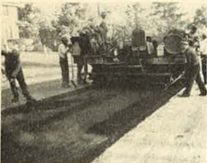
FIG. 7.—Spreading 1\frac{1}{2} in. plant mix bituminous concrete on an old bituminous road with a paving machine to level and strengthen the old surface.
