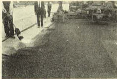
FIG. 3.—Warming an old surface to make a feather edge joint at junction with new pavement.
