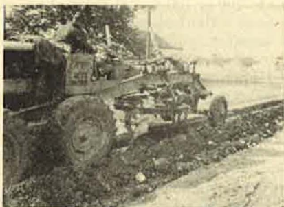
FIG. 8.—Excavating the narrow trench along the old pavement with specially designed grader blade, etc.
