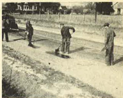
FIG. 2.—Making a paint patch; bitumen applied from a hose is spread with a broom, covered with fine aggregate and rolled.
