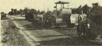
FIG. 6.—Making a road mix of open graded aggregate and a heavy bitumen by once over with the mixing machinery, etc.
