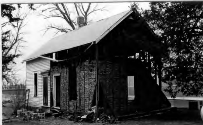
Left: Double-pen house with brick nogging is north of Concordia in Freedom Township. Other examples of houses with brick nogging were found in Concordia.
