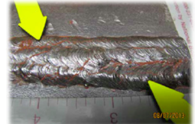
Figure 3. SCC on weld cap with Visible MT (red).
