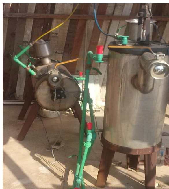
Fig. 2. The biogas digester are horizontal and vertical shape
