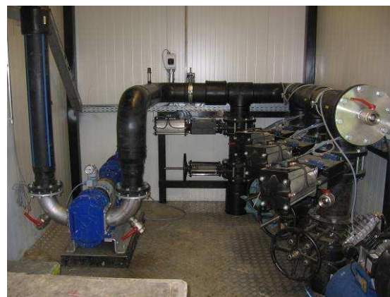
Fig.3. Pumping station in a biogas plant [1]
