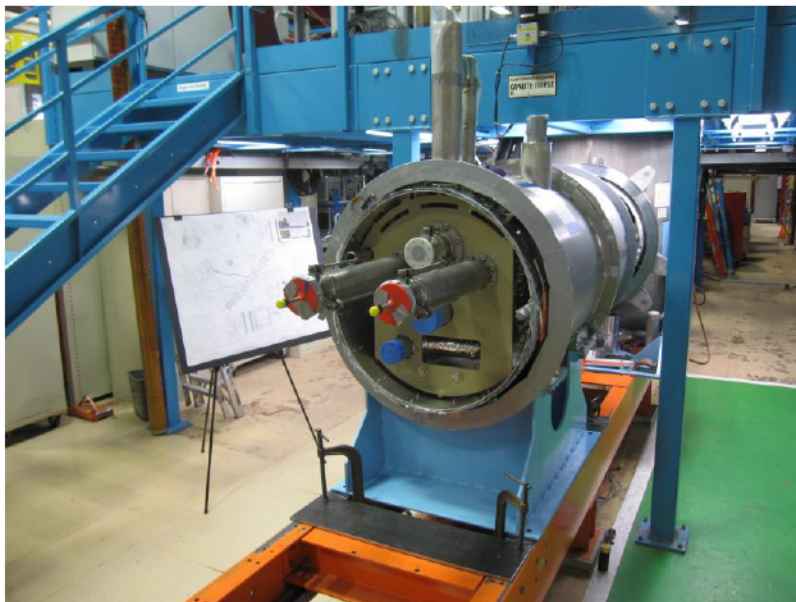
Figure 77: New Adapter Box with a thermal shield between the feed can and the Cryo-Assembly.
