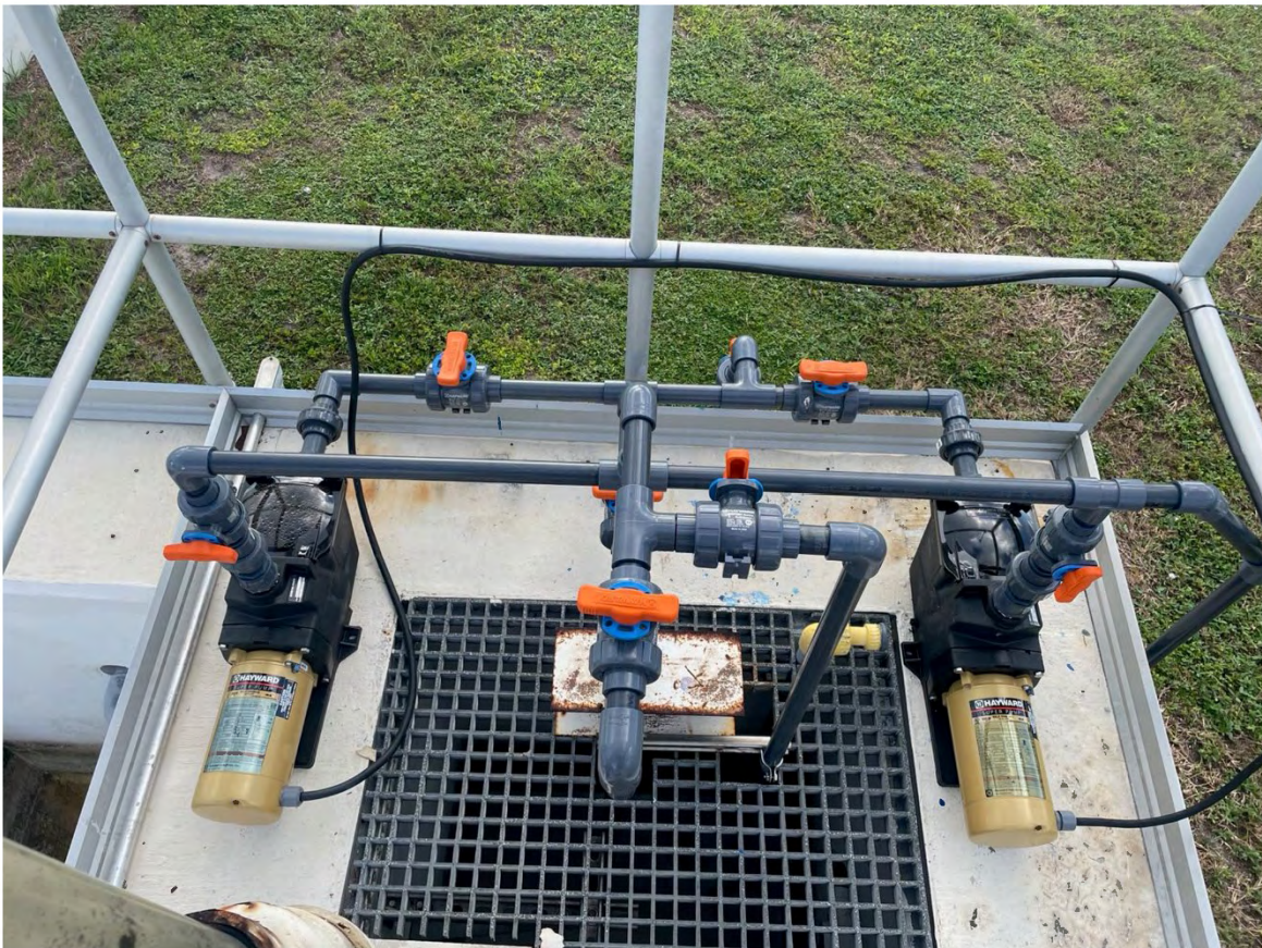
Filtered Effluent TSS Sample Pumps
