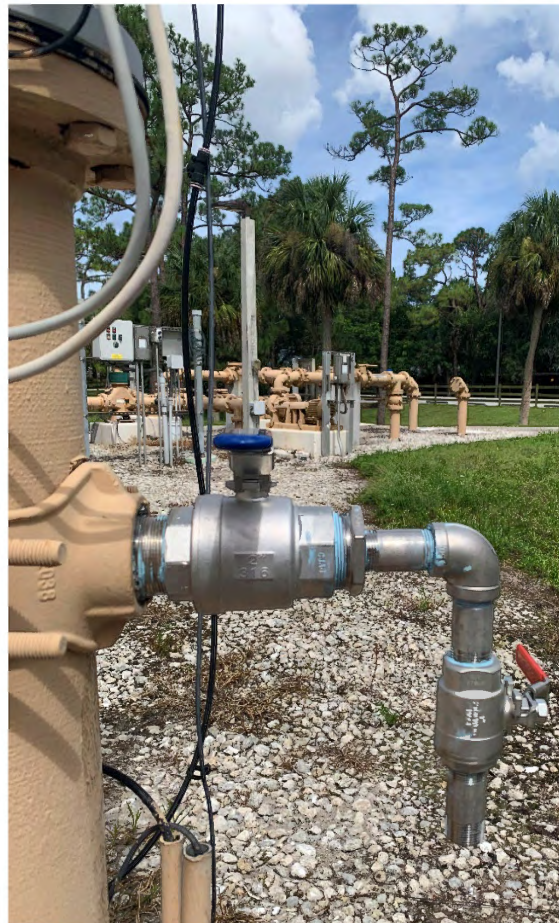
Replacement WAS Sample Port
