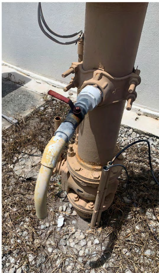
Existing WAS Sample Port
