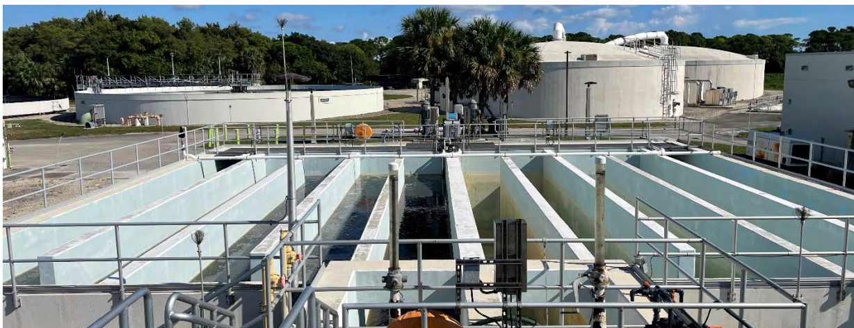
Chlorine Contact Disinfection Chambers
