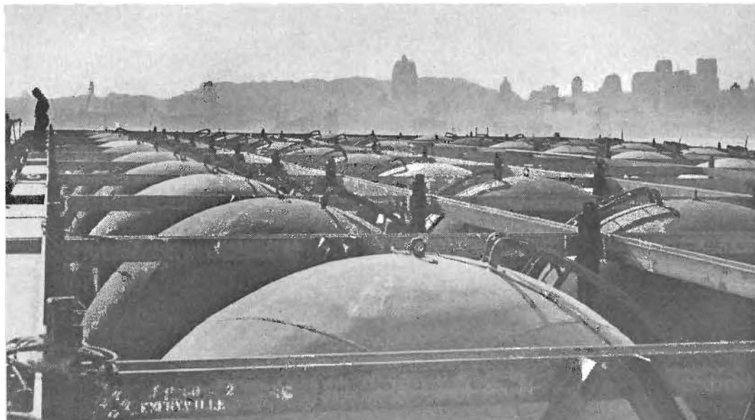
DOMES OF STEEL forming the tops of the 55 cylinders in the world's largest compressed air flotation caisson for the concrete center anchorage of the San Francisco-Oakland Bay Bridge are shown in the above photograph revealing San Francisco's skyline in the background as the caisson is being sunk in mid-bay. The domes are alternately cut off and rewelded into place as the cylinders are increased in height. The caisson is 92 feet wide by 197 feet long and the anchorage when completed will be 478½ feet high and project 298½ feet above water.
