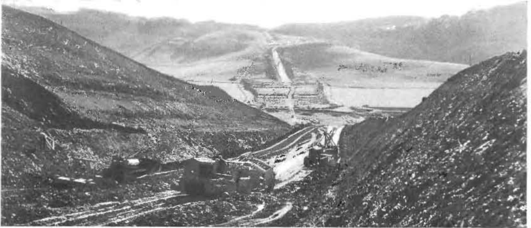
"BIG FILL," adjacent to the "Big Cut," is 2500 feet long, with a maximum height of 75 feet, requiring 605,600 cubic yards of material.
