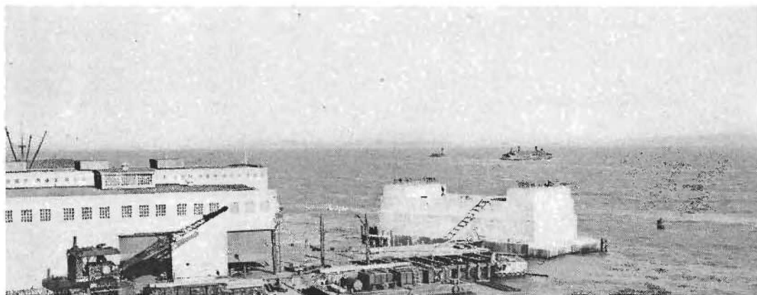
UP FROM THE DEPTHS of the bay off the end of San Francisco's Harbor Dock No. 24 a mass of solid concrete the size of a 7-story building has been constructed from bedrock to a height of 40 feet above water. It constitutes Bridge Pier No. 2 and is all ready for the great steel tower that will be erected upon it.
