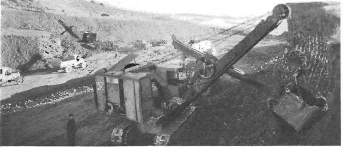
"BIG CUT" of the American Canyon cut-off project where a total of 520,500 cubic yards will be moved. The cut is 2400 feet long with 130-foot maximum depth.
