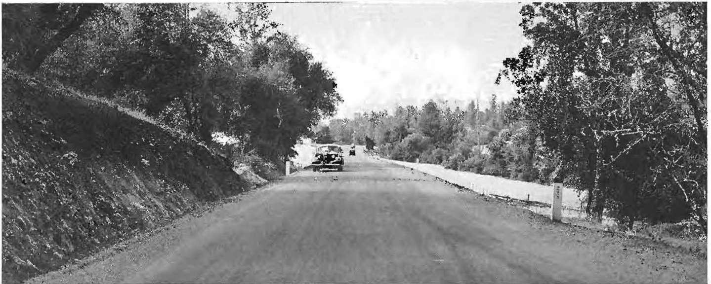
Construction of realigned highway between Parks Bar Bridge and point one-fourth mile east of Nevada County line eliminated such poor alignment as shown in upper photograph. Center—Showing how new highway approaches bridge with safe sight distance and curve. Lower—Section of newly completed highway.
