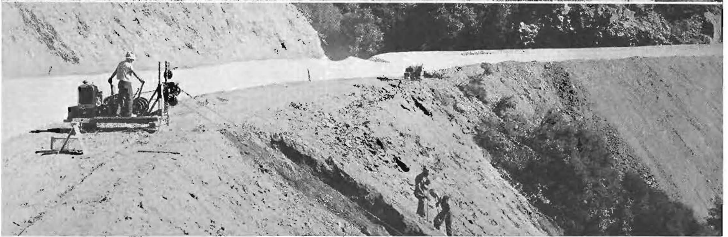
Scenes on Angeles Crest Highway. Upper—Section of new highway showing erosion control treatment applied to fill slopes. Center—Typical grading operations on highway near Chilao, ten miles northeast of Red Box. Lower—Illustrating method of flattening fill slopes prior to applying erosion control treatment.
