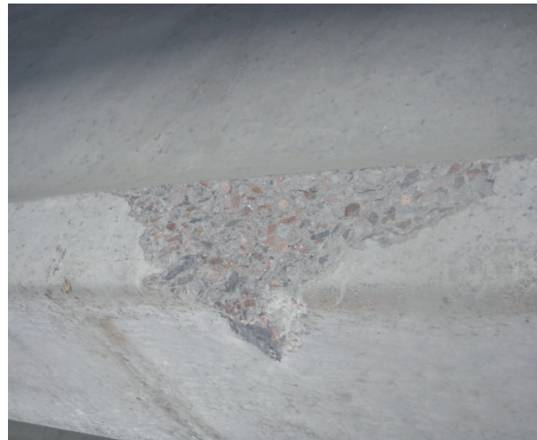
Figure 11 Damage of the protective concrete cover in the widened lower part of beam No. 7 from the Kapshagai side
