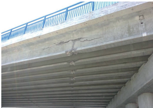
Figure 3 A general view of the destruction in beam No. 1 from the Kapshagai side (Destruction of the bottom flange of beam and its widened lower part. A longitudinal crack was revealed in the upper part of the beam flange of a length of about 8.6 m)
