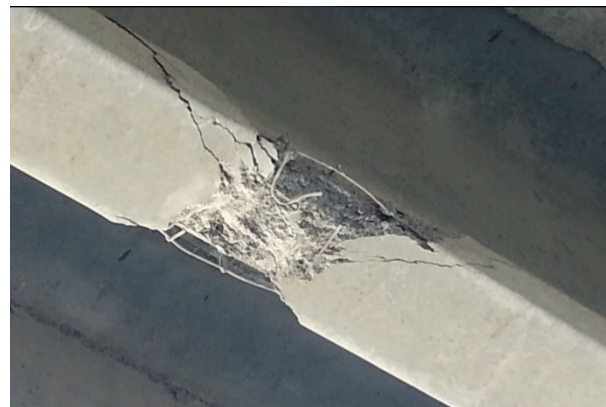
Figure 5 A general view of the destruction of the bottom flange of the beam No. 2 (The reinforcement of the smooth and periodic profile is damaged. The bundle of prestressed reinforcement is exposed)
