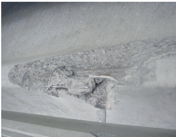
Figure 9 Fragment of the destroyed widened lower part of beam No. 5 from the Kapshagai side (The reinforcement is torn; the bundle of prestressing reinforcement is exposed)
