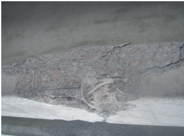
Figure 8 Destruction of the widened lower part of the beam No. 11 from the Kapshagai side (The reinforcement of the smooth and periodic profile is damaged. A longitudinal crack was revealed in the upper part of the beam rib of a length of about 3.9 m)
