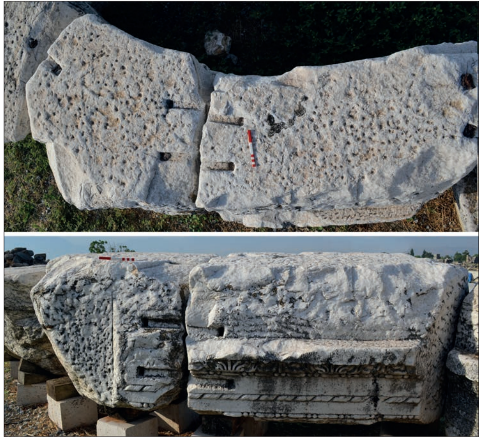
10. - Theatre, second order: upper and rear face of a frieze-architrave repaired during the 4 th cent. AD restoration of the scaenae frons.
