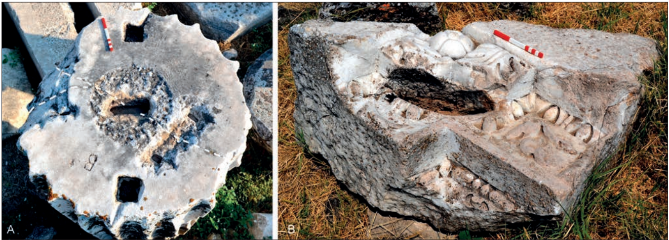
5. - Sanctuary of Apollo, Temple B, drum with cramps used to repair a crack (A); Nymphaeum of the Tritons, cornice with a natural cavity that was reshaped to hold a replacement part (B).
