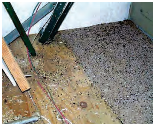
Figure 4. Heavy rodent contamination.
