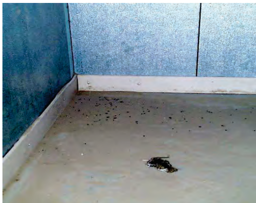
Figure 3. Light rodent contamination.
