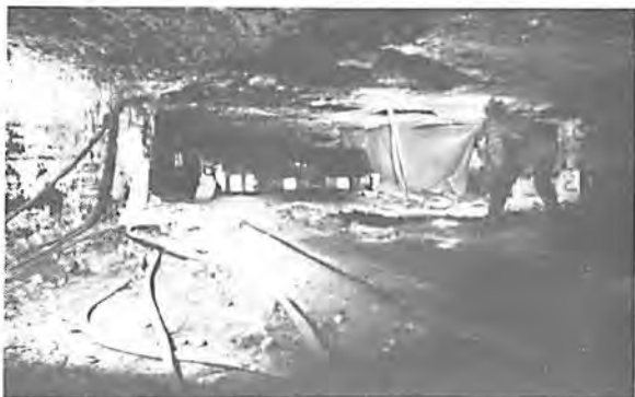
Multiple flash photo of a face lobby showing the complex network of power cables necessary, with Laribee's Bob Ogden and a shuttle car in the rear.
