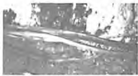
Power cables make a 230° turn around a pillar. Cable at bottom (being replaced) shows the terrific stresses a mine cable must undergo, and still perform reliably.
