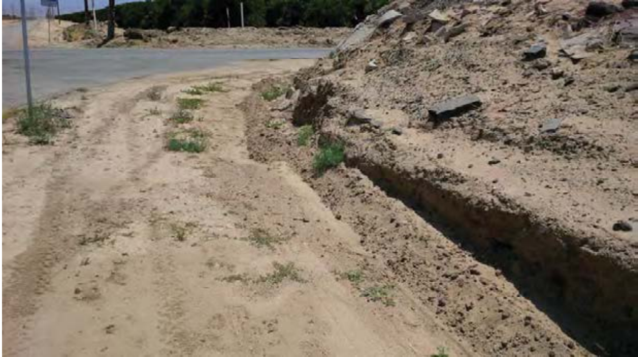
Photograph 6: Project: Bena Sanitary Landfill (SPK-2014-00236) Taken By: James Robb, USACE Date: May 8, 2014
