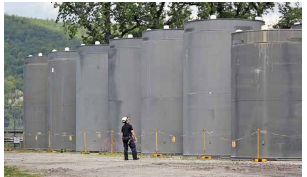
These casks are used to store spent fuel rods at Indian Point. Photo by John Meore/The Journal News
