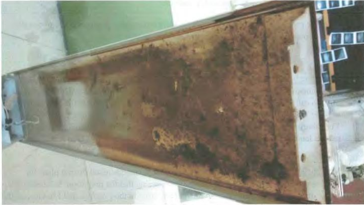
6 7 8 9 10 11 12 13 14 15 16 17 Figure 1: Ballast leak in Room C (Note: photo taken April 2014, tray replaced May 2016)
