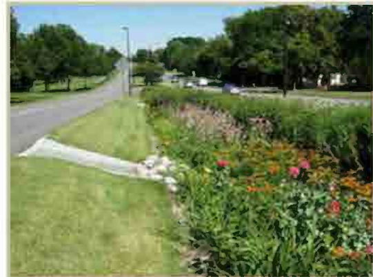
Typical bioswale with directed drainage from roadway as per Soil Science Society.
