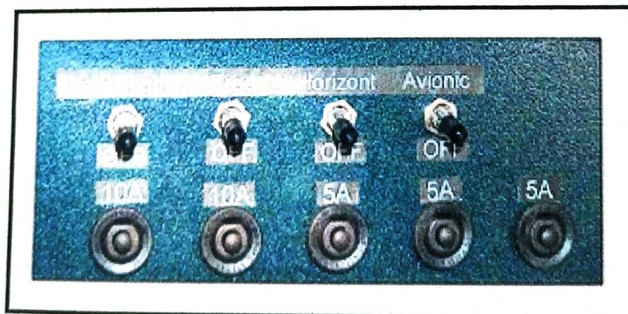
Figure 7 – Switches and fuses panel
