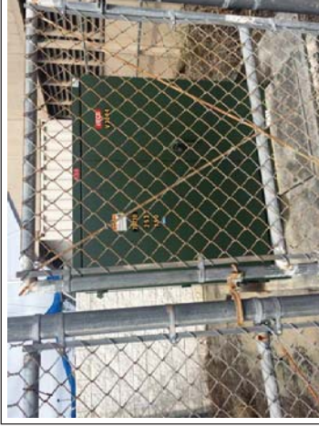
Photograph 25: HECO transformer that appeared to be in good condition.
