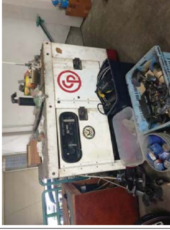
Photograph 19: SOEST / METC generator with diesel tank.
