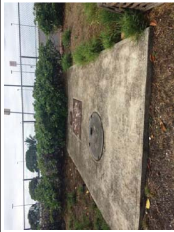
Photograph 22: Oil water separator and underground storage tank.
