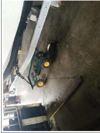
Photograph 23: Floor drains in the maintenance shop that lead to the oil water separator.
