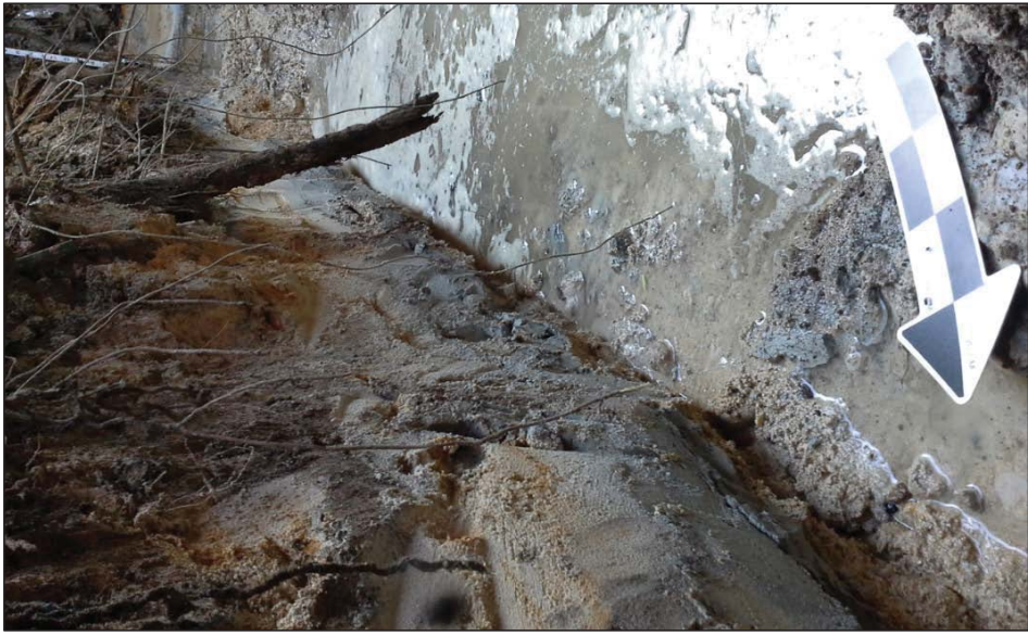
Figure 54. T-7 northeast sidewall profile close-up at the base of excavation, view to east to the BOE
