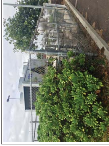
Photograph 26: SOEST / METC air conditioning unit.
