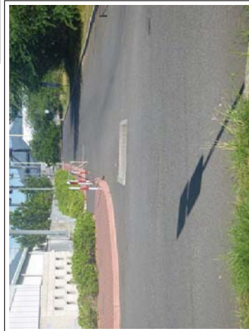
Photograph 24: Storm drain at entrance to the SOEST / METC facility.
