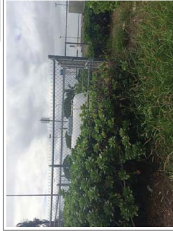
Photograph 27: SOEST / METC propane tank.
