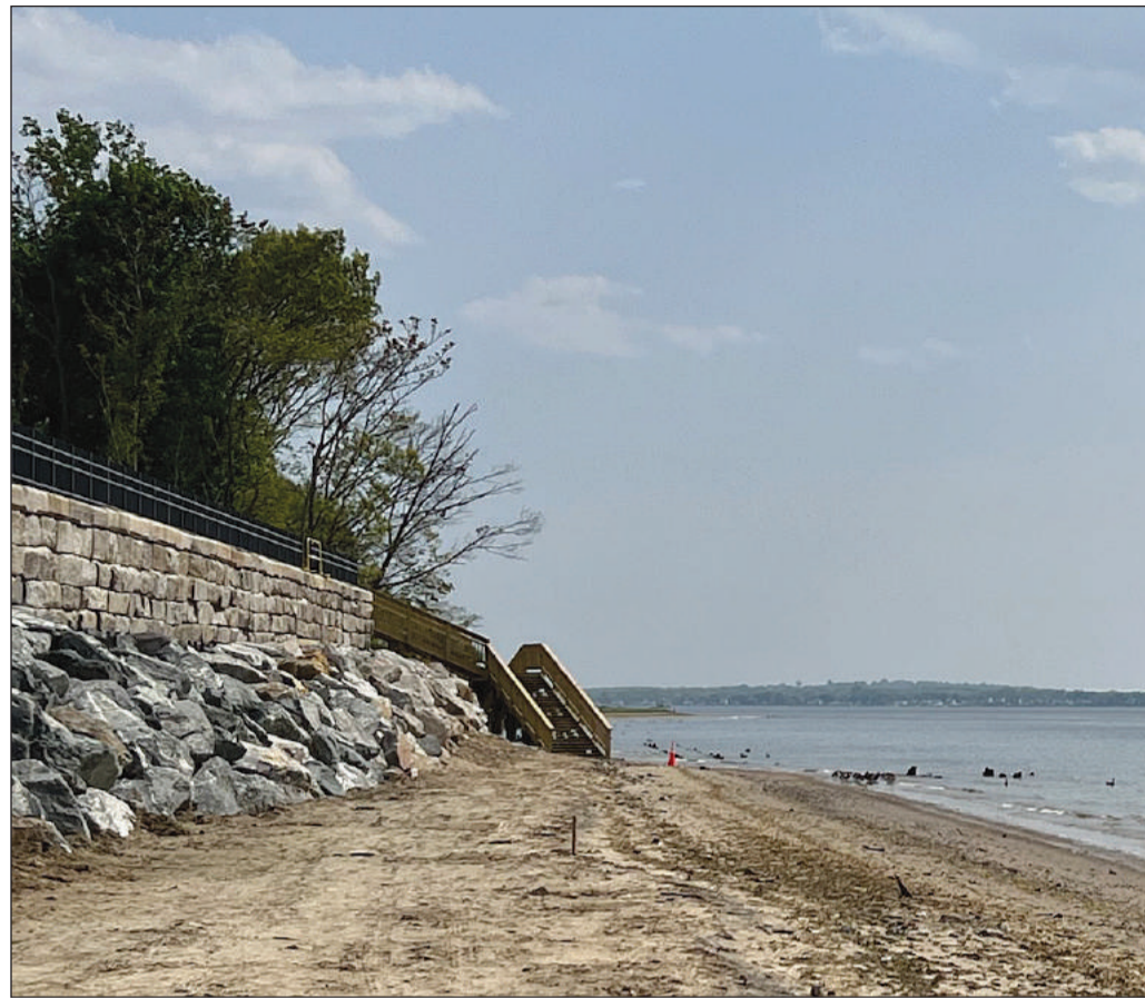
A look down the reconstructed seawall at Crescent Park towards the bluffs that will also be refurbished after the city recently gained a Rhode Island Infrastructure Bank grant.
