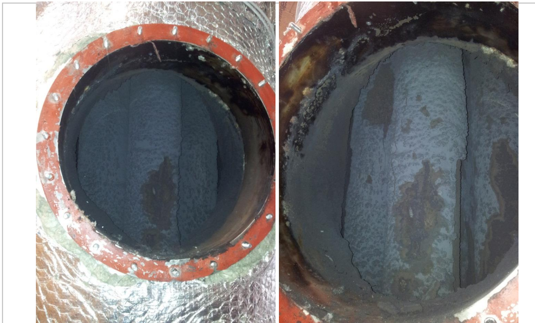
Figure 17: Left: Filters before pulse blow. Right: Filters after 3 pulse blows
