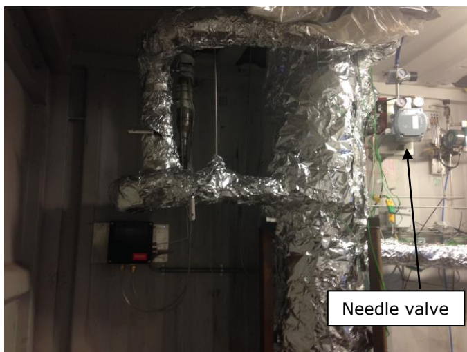
Figure 52: System inlet (left), filtration unit (middle) and needle valve (right)
