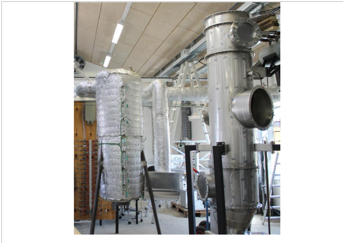
Figure 11: Spray cooler (left) and filter house (right) prepared for tracing
