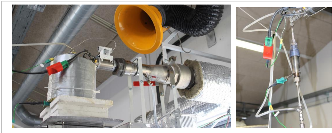
Figure 13: Left: Hot gas filter probe installation - Right: Connection for hot gas filter probe
