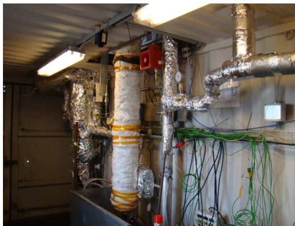
Figure 53: Filtration unit (left), reactor (middle) and system outlet (right)
