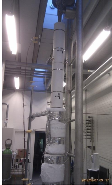
Figure 48: Pilot reactor with visible heating elements.
