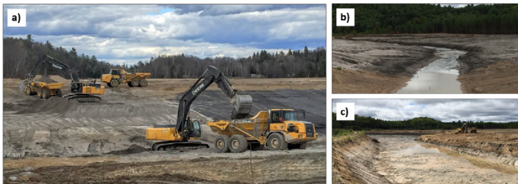
Figure 5 Photos showing the central drainage channel excavation: a) tailings for paste feedstock being loaded into rock trucks for hauling to the TMA-1 stockpiles; b) downstream section of the excavated central drainage channel where tailings grain size is relatively coarse; c) upstream section of the excavated drainage channel where the tailings grain size is relatively fine
