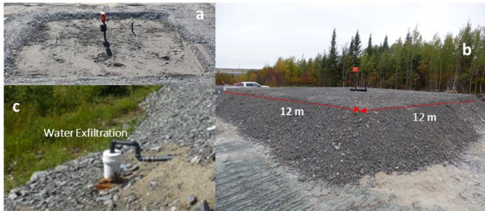
Figure 3 Final profile of the control cell (a), CCBE experimental cell (b) and exfiltration waters (c)
