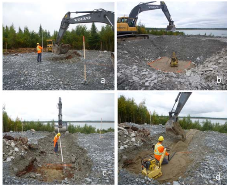
Figure 1 Excavation with a hydraulic excavator (a), inverted truncated pyramid form of the experimental cell (b), excavation of the trench (c) and installation of the PVC pipe for water exfiltration (d)
