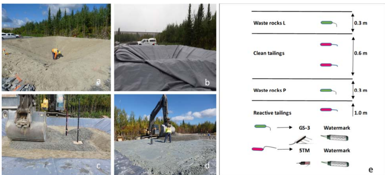
Figure 2 Sand and geomembrane setting up (a and b), sensor placement and setting up the different layers of the field experimental cell (c and d) and location of the instruments in the cover (e)
