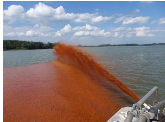
Figure 13 In-lake treatment with a dry iron product at the artificial reservoir Quitzdorf
