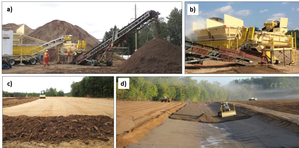
Figure 4 Photos showing the cover material construction methodology: a) overview of pugmill mixing equipment and stacker creating a daily stockpile of SGB material; b) close-up of the hopper and pugmill mixing equipment; c) spreading and compacting SGB material; d) spreading erosion protection within a drainage swale using a GPS-guided dozer
