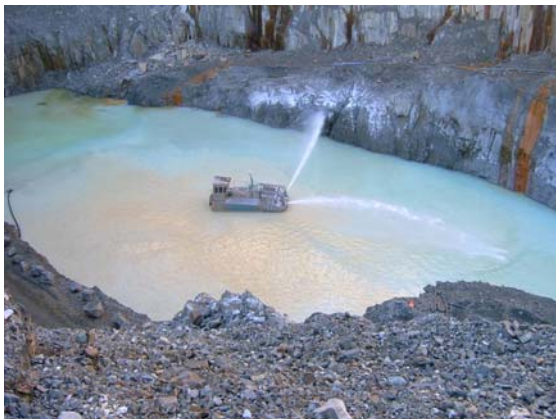
Figure 10 Aerial photo showing the distribution of lime above the surface, AMD treatment, North Sweden
