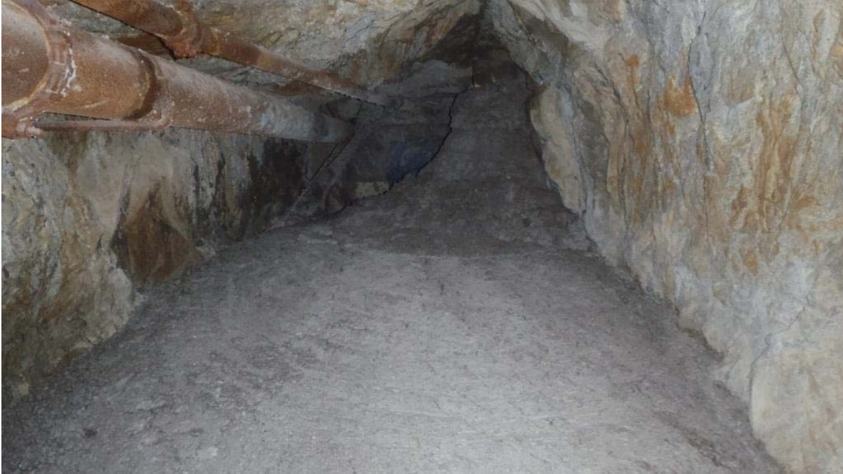
Figure 3 Paste barricade mix delivered via borehole to plug the door to the shaft
