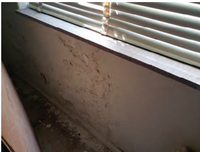
Fig-9 Damaged sill wall with electrical outlet
