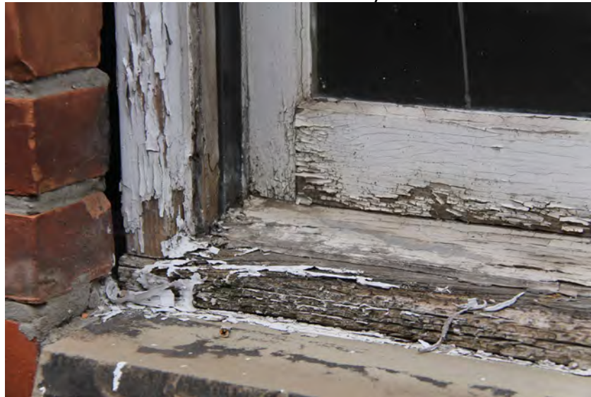
WINDOW #H3 ROTTED SILL
