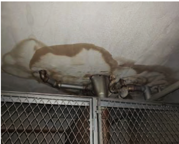
Fig-6 Water-damaged plaster ceiling in locker room
