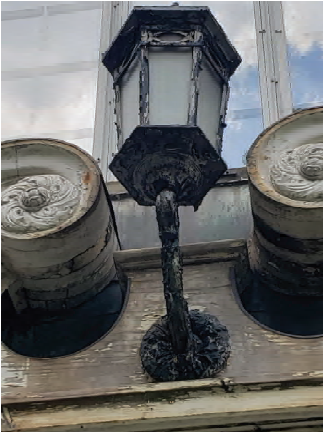
Fig-34 Historic light fixture with flaking paint and possible corrosion.
