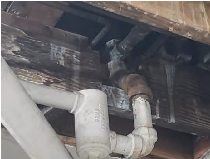
Fig-29 Damaged joist at mechanical room piping
