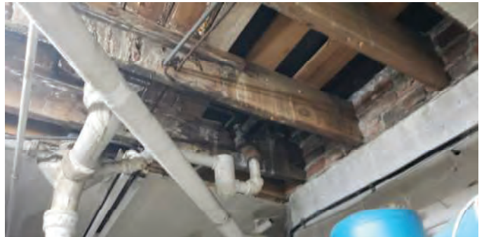
Fig-24 Mechanical room water damage. Sister water damaged joist.
