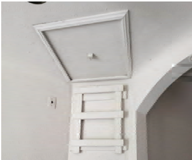
Fig-11 Attic access hatch is directly adjacent to stair landing.
