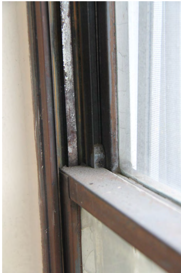
WINDOW #U19 INTERIOR RUSTED BALANCE TAPE TYPICAL
