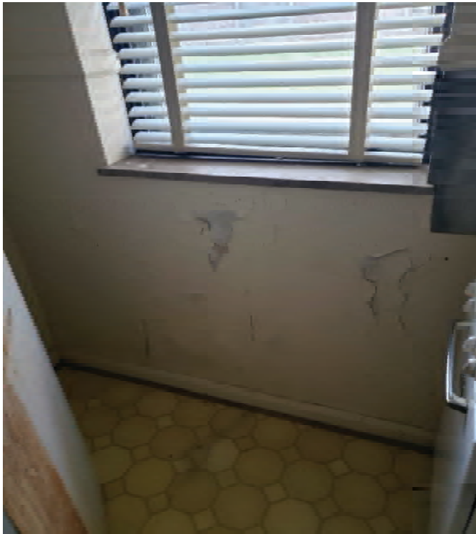
Fig-8 Damaged sill wall
