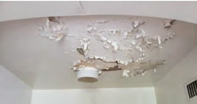
Fig-22 Apartment 209 kitchen ceiling water damage
