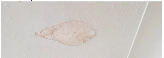
Fig-25 Ceiling water damage. Remove to expose existing structure.
