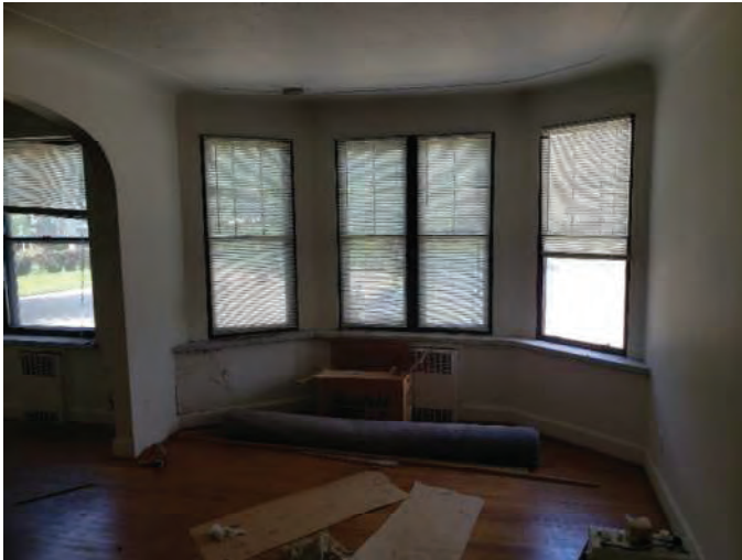
Fig-26 Water damage at corner of bay window matches exterior repointing.
