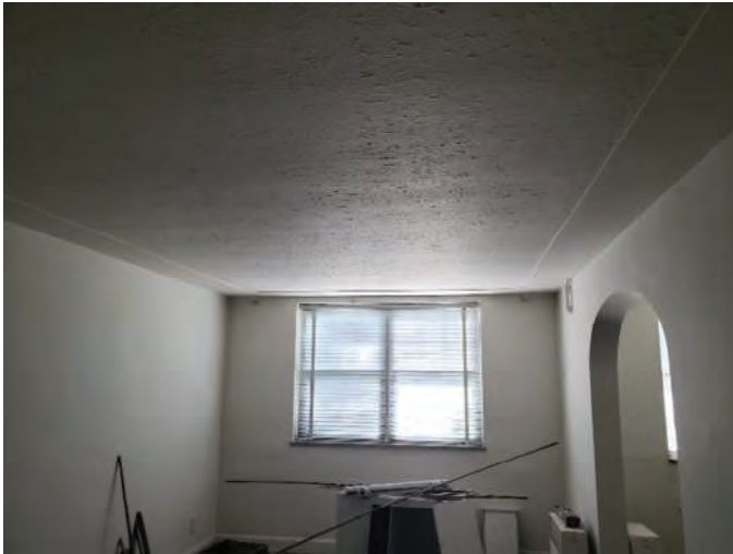
Fig-30 Water damage at window ac units
