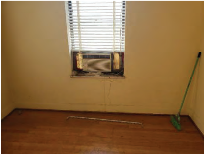
Fig-28 Water damage at window ac units
