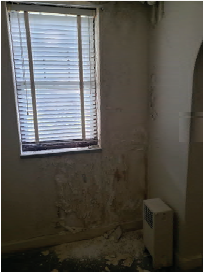
Fig-19 Damage plaster at semibasement
