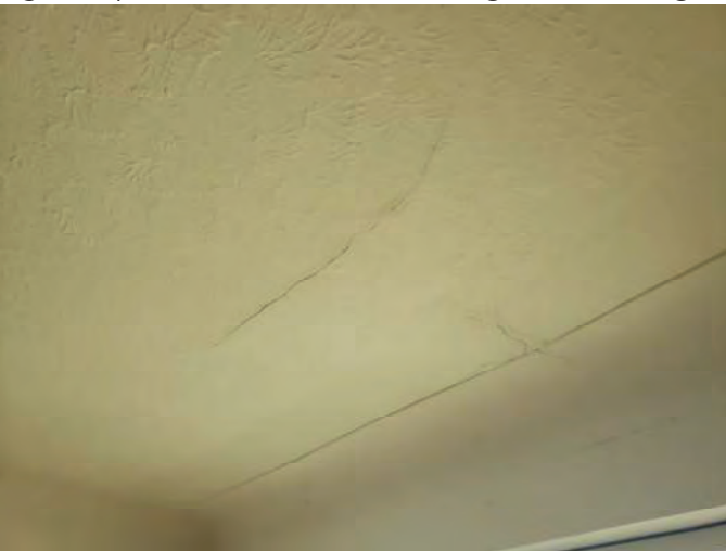
Fig-23 Apartment 209 living room damage
