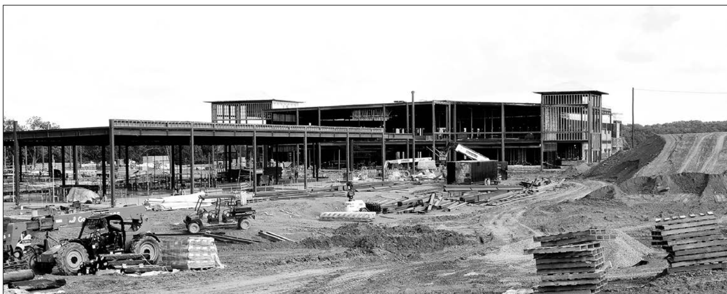
Cartersville Primary School's new building is situated on Carter Grove Road in the Carter Grove subdivision and will feature three playgrounds.
