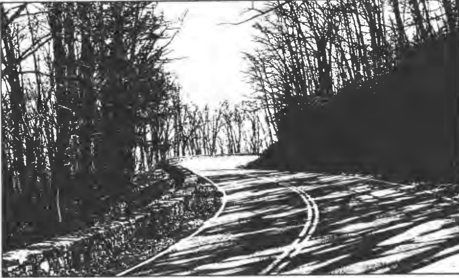
A 75-mile portion of Skyline Drive at Shenandoah National Park overlooking the Blue Ridge Mountains of Virginia required the rehabilitation of a 22"-high, dry-laid stone wall [opposite]. The new wall was built to a height of 27" whereas code normally requires a height of 36". The wall was constructed of precast concrete, clad with split stone and mortar joints [center]. To achieve visual compatibility, recessed mortar joints were arranged in a random pattern [bottom]. (courtesy NPS and Paul Daniel Mariott)
