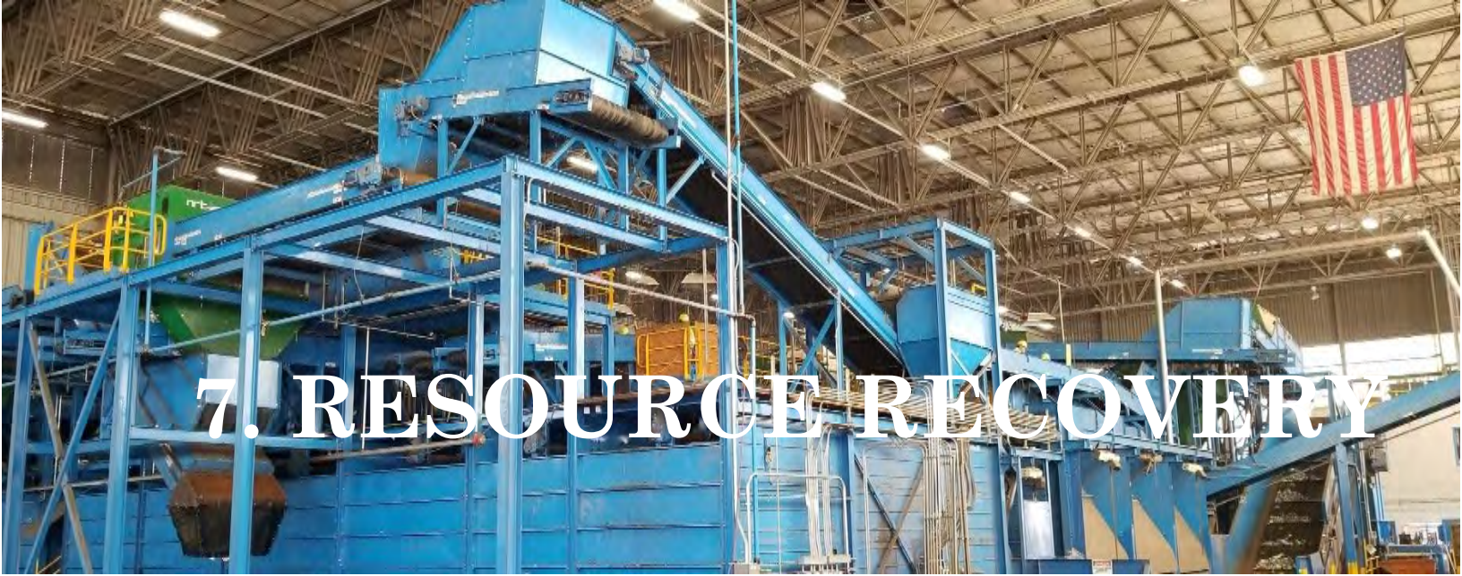
Milwaukee's Materials Recovery Facility
