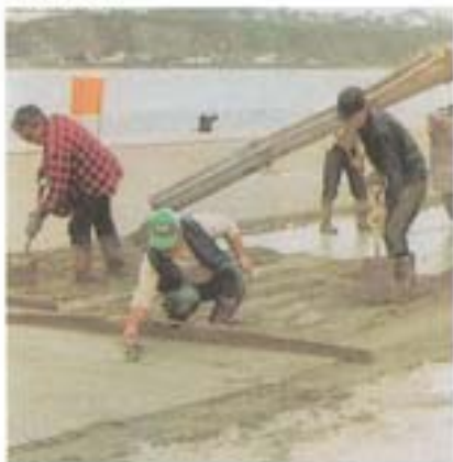
Concrete modified with PLANICRETE in the Old Port of Quebec City, Canada
