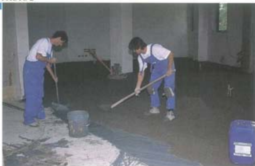
Preparing a screed at the headquarters of Colnago Bicycles outside of Milan, Italy
