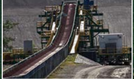
At the end of the static conveyor, the overburden is transferred to a computer-controlled "crawling" spreader arm
