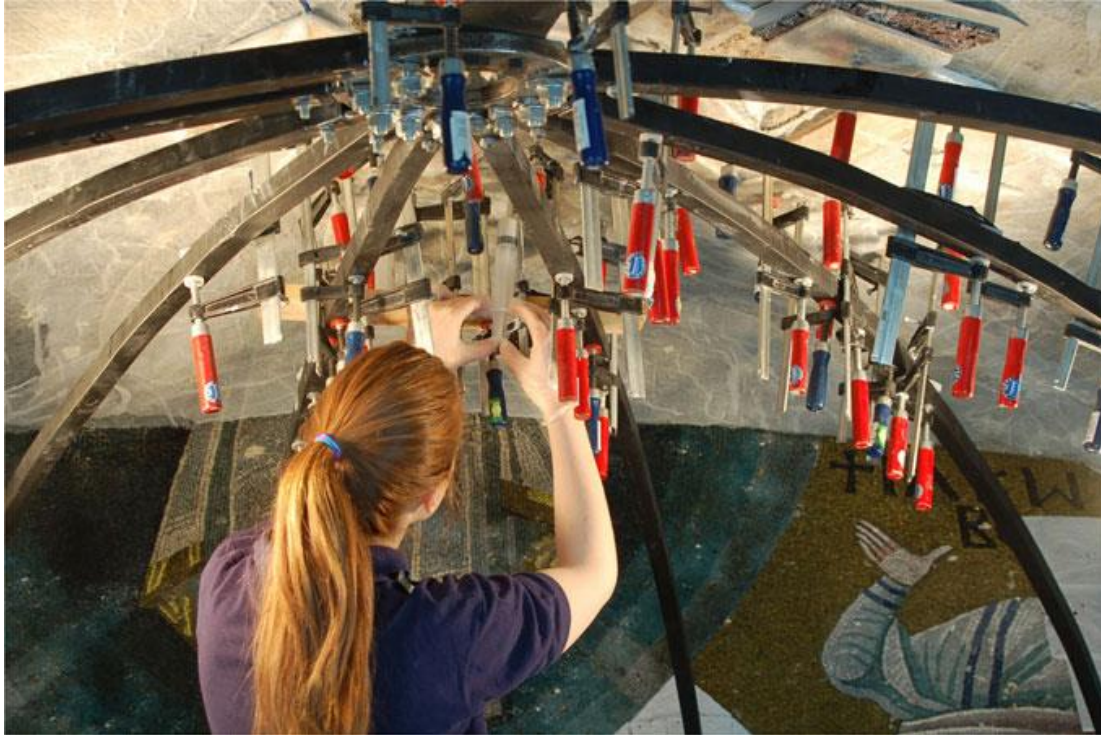
Illustration 6. The metal structure (the “spider”) supporting the mosaic in the apse during consolidation (Foto Araldo De Luca - CCA)
