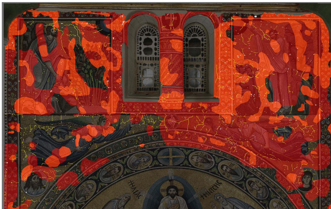
Illustration 2. Graphic documentation of mosaic detachments from the wall of the main arch. In red the surfaces completely detached.
