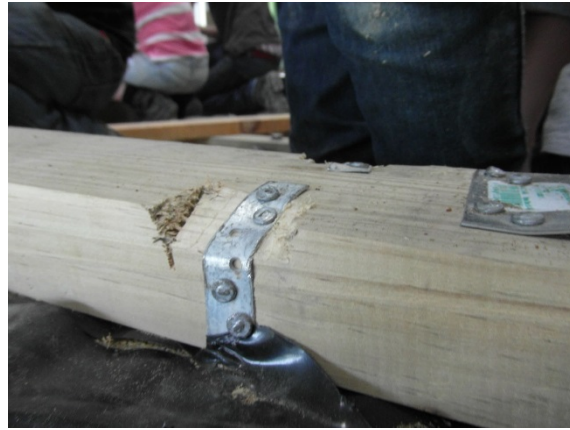
Figure 65: Photo of sole plate fixed to upstand with cast-in off-the-shelf steel straps, after nailing
