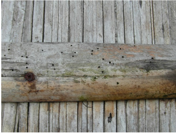
Figure 30: Beetle damage in bamboo, Ecuador – exit holes are clearly visible (Kaminski, 2016)
