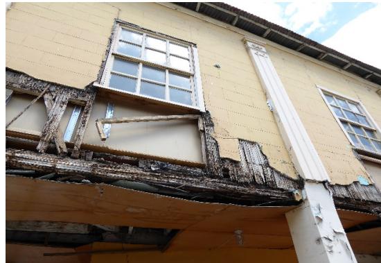
Figure 43: Rot (and possibly termite) damage to traditional bahareque housing, Ecuador (Kaminski, 2016)
