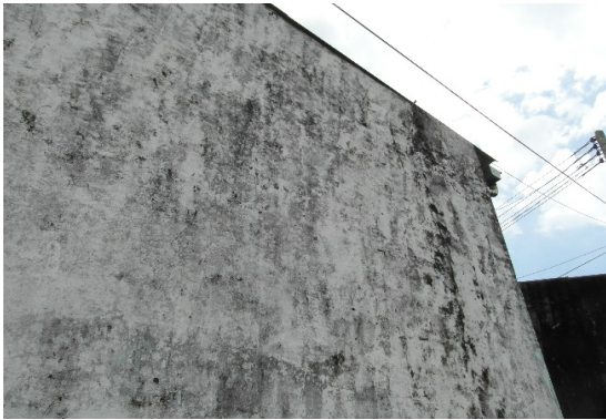
Figure 42: Engineered bahareque house in Colombia with no roof overhang – the mould on the wall is clearly visible (Kaminski, 2016)
