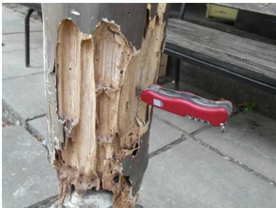
Figure 34: Severe termite damage in bamboo, Costa Rica. Note how the outer painted silica shell of the bamboo is still intact in some areas and hence appears in good condition (Kaminski, 2016)
