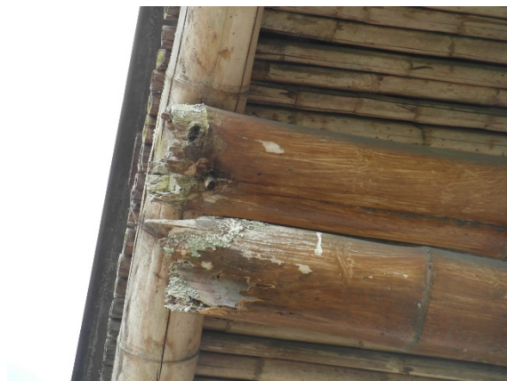
Figure 39: Rot to the exposed end of the bamboo in a roof, Costa Rica (Kaminski, 2016)
