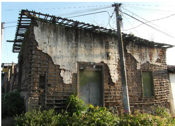
Figure 3: Traditional bahareque housing in Berlín, El Salvador. The outer render has spalled off (Kaminski, 2016)
