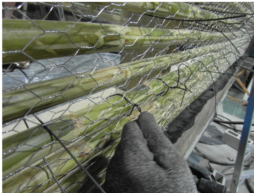
Figure 72: Installing steel wire through-ties to connect chicken mesh on both sides of the matrix
