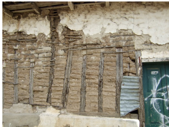
Figure 33: Severe termite damage to timber and cane in traditional bahareque, El Salvador (Kaminski, 2016)
