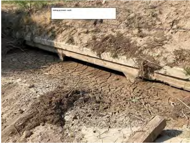
Figure 28: Impacted Box Culverts
