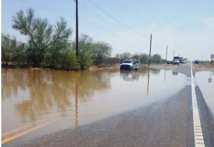
Figure 58: MP 43.58 Roadway Flooding and Closure 2018 (Picture Provided by ADOT)
