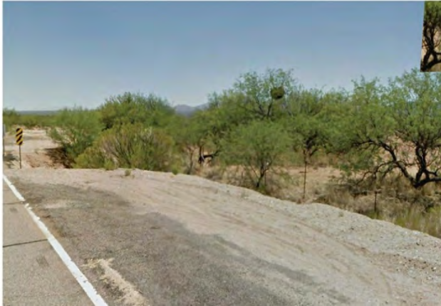
Figure 81: Northbound SR286 shoulder conditions (2011) facing northeast
