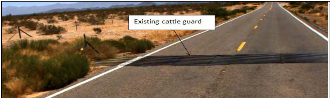
Figure 21. Existing Cattle Guard at MP 24.21
