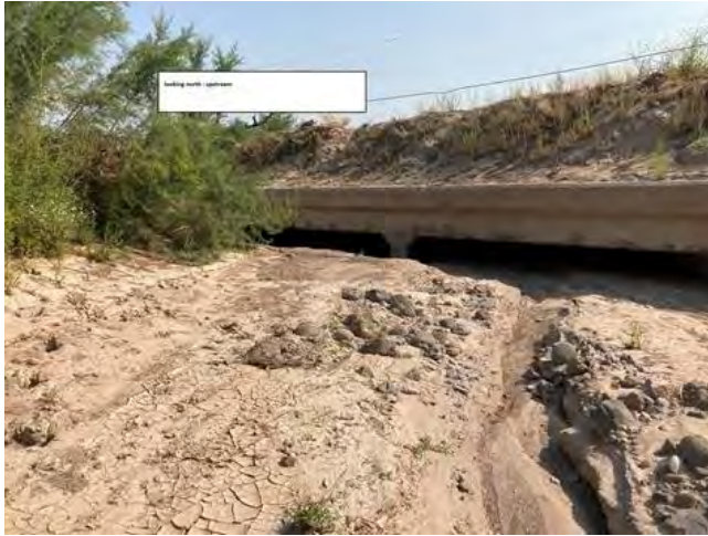
Figure 25: Impacted Box Culverts
