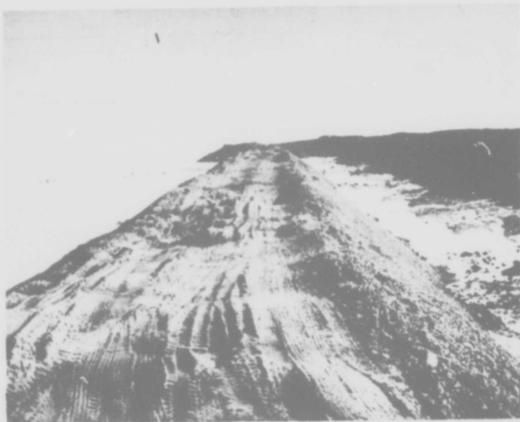
Figure 17. Surface of crushed rock test section after two thaw seasons, 11 August 1959.
