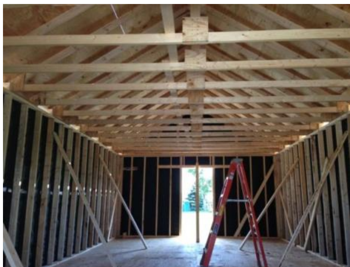
Figure 2-6. Interior view of the Enhanced Shelter and the installation of the wall felt air barrier.
