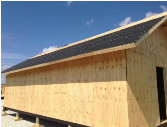
Figure 2-2. Exterior view of the Enhanced Shelter showing the roof and floor (at the rim joist) felt air barrier.
