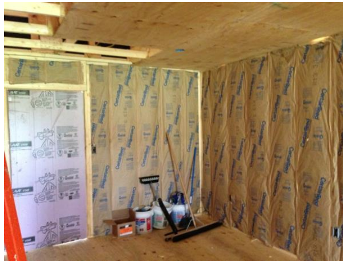
Figure 2-7. Interior view of the Enhanced Shelter showing the wall and door insulation applications.
