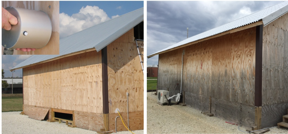
Figure 4-6. Discoloration of the exterior walls (left new, right after 20 months) and wide variation in SR on the same side of the wall (as evidenced by the color difference).
