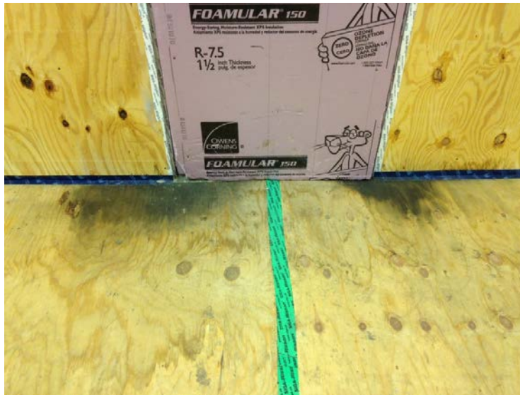
Figure 5-3. Entry of enhanced B-hut showing water stains and mold from entry of rainwater.
