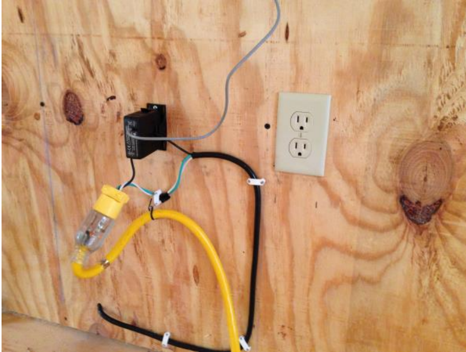
Figure 3-3. Control Shelter transducer clamp attached to the HVAC power cable.
