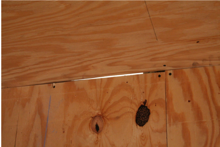
Figure 5-1. Gap in ceiling/wall connection as shown by light entering the space.
