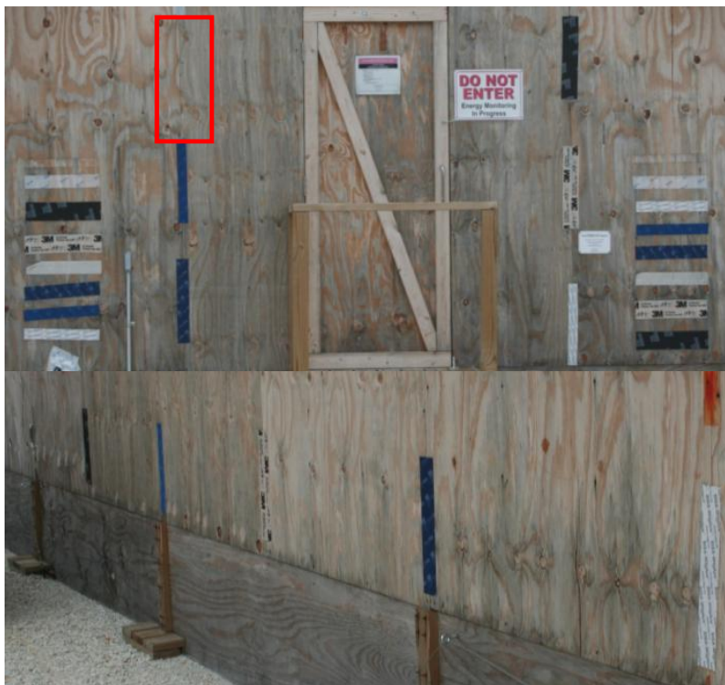
Figure 2-18. Outdoor Weathering Samples after 8 Months: Approximately 8 months after application (28 May 2014) on the south wall (top) and west wall (bottom). Tape D in the vertical W location (indicated with the red box), completely peeled off within the first 2 months.
