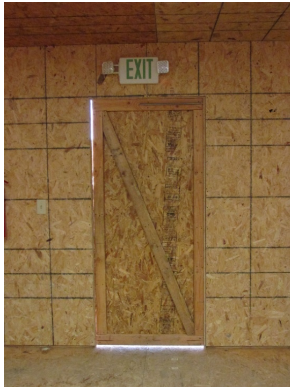
Figure 5-2. Typical B-hut leaky door.
