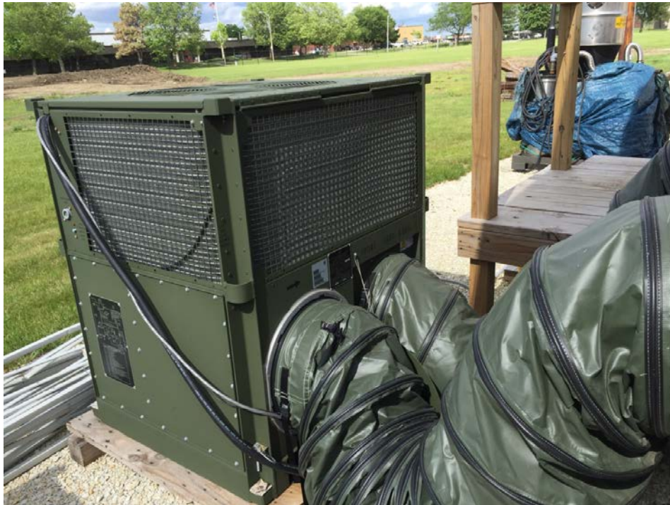
Figure 4-45. IECU serving the B-hut and the flexible ducts used as supply and return ducts.
