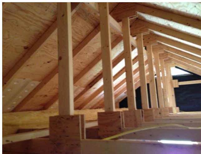
Figure 2-8. View of attic insulation and baffles in the Enhanced Shelter.
