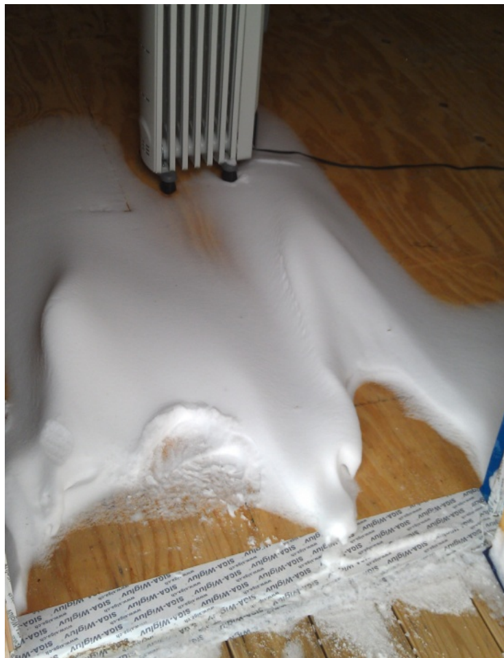
Figure 5-4. Snow blown in under sill of B-hut door.
