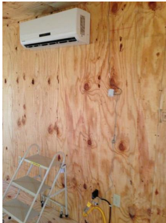
Figure 3-2. Placement of the Control Shelter's metering equipment.
