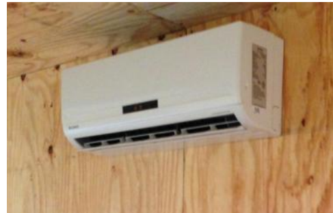
Figure 2-3. Chigo mini-split interior AHU.
