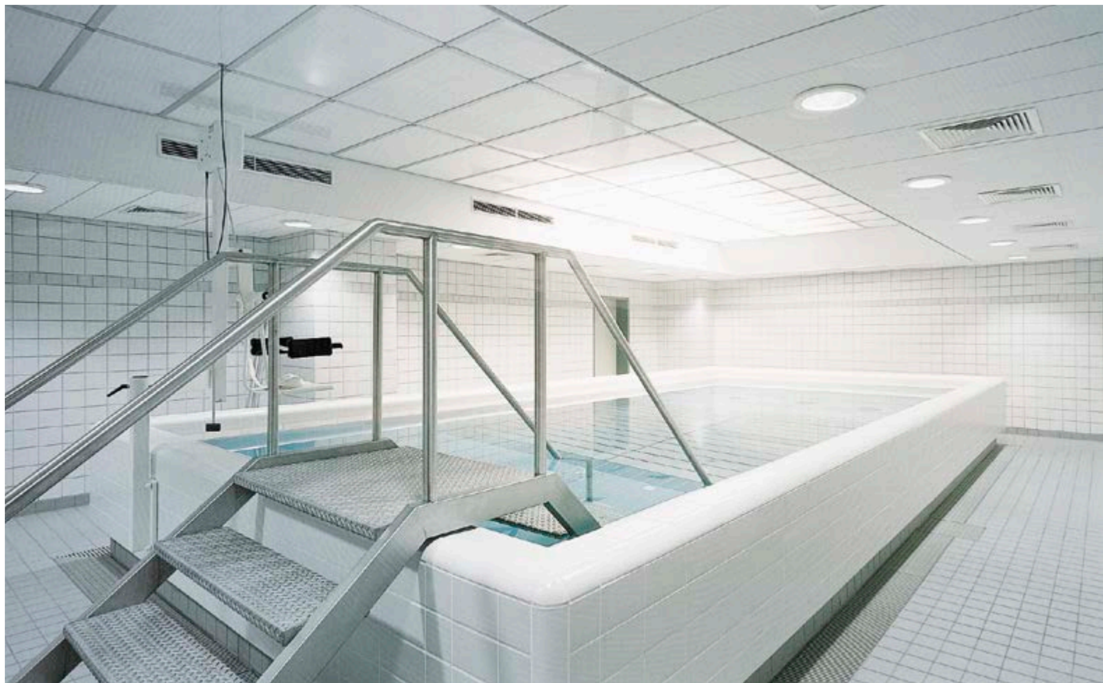
More hygiene in nursing and therapy areas Krankenhaus der Barmherzigen Brüder, Munich, Germany / Architect: H. Kochta & Partner, Schirmer & Schrader / Photo: Monika Custodis
