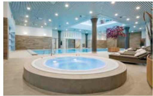
Sustainably effective and practical for pools Okura Hotel Amsterdam, Netherlands / Photo: Marcel van der Burg
