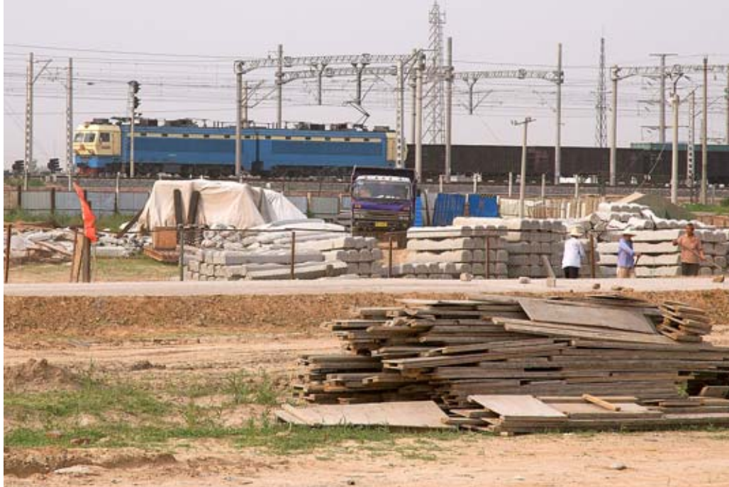
In June 2009, an electric-hauled freight passes an intermodal yard under construction in Zhengzhou, a crossroads for China's main east-west and north-south rail lines. George W. Hamlin
