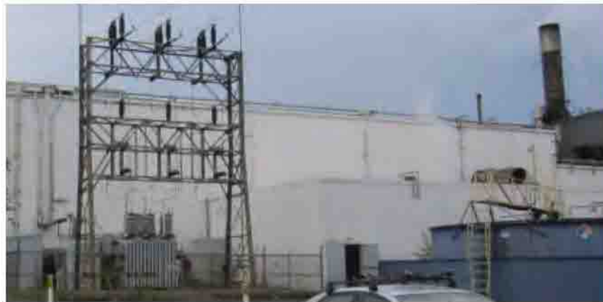
Figure 1 – Main Transformer (Boiler Stack in Background)
